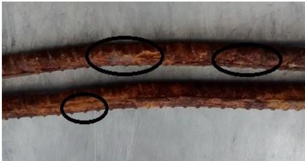
Figure 4.8: Pitting corrosion in the tensile bars of beam B4
