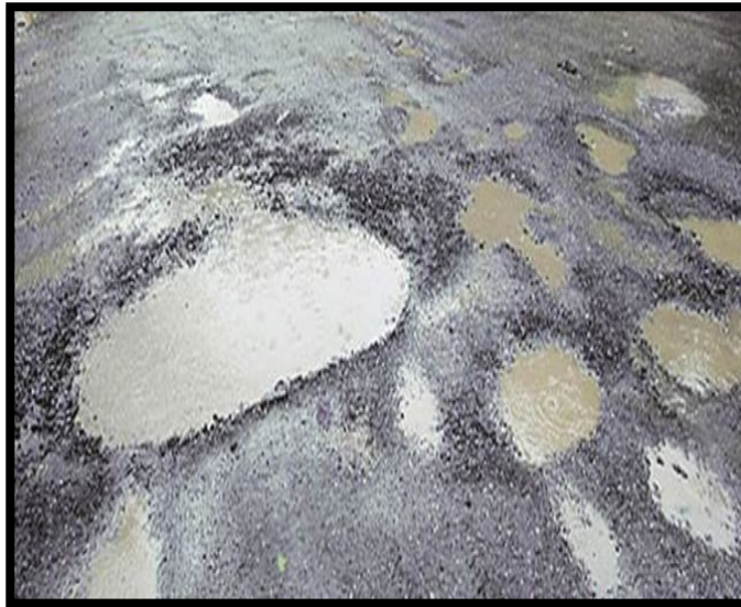
b) Moisture Induced Damage (Stripping) at Field
