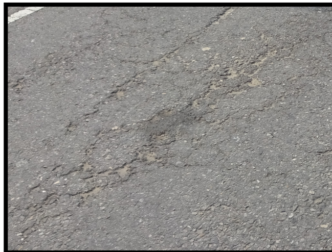
b) Fatigue cracking failure
