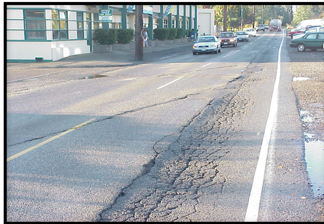
a) Rutting type of field failure
