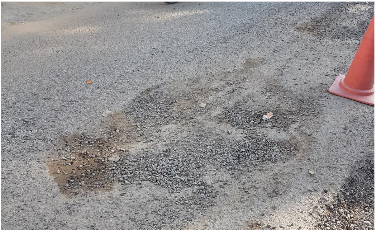
Figure 4.9: Large Ravelled Area at Section DN
