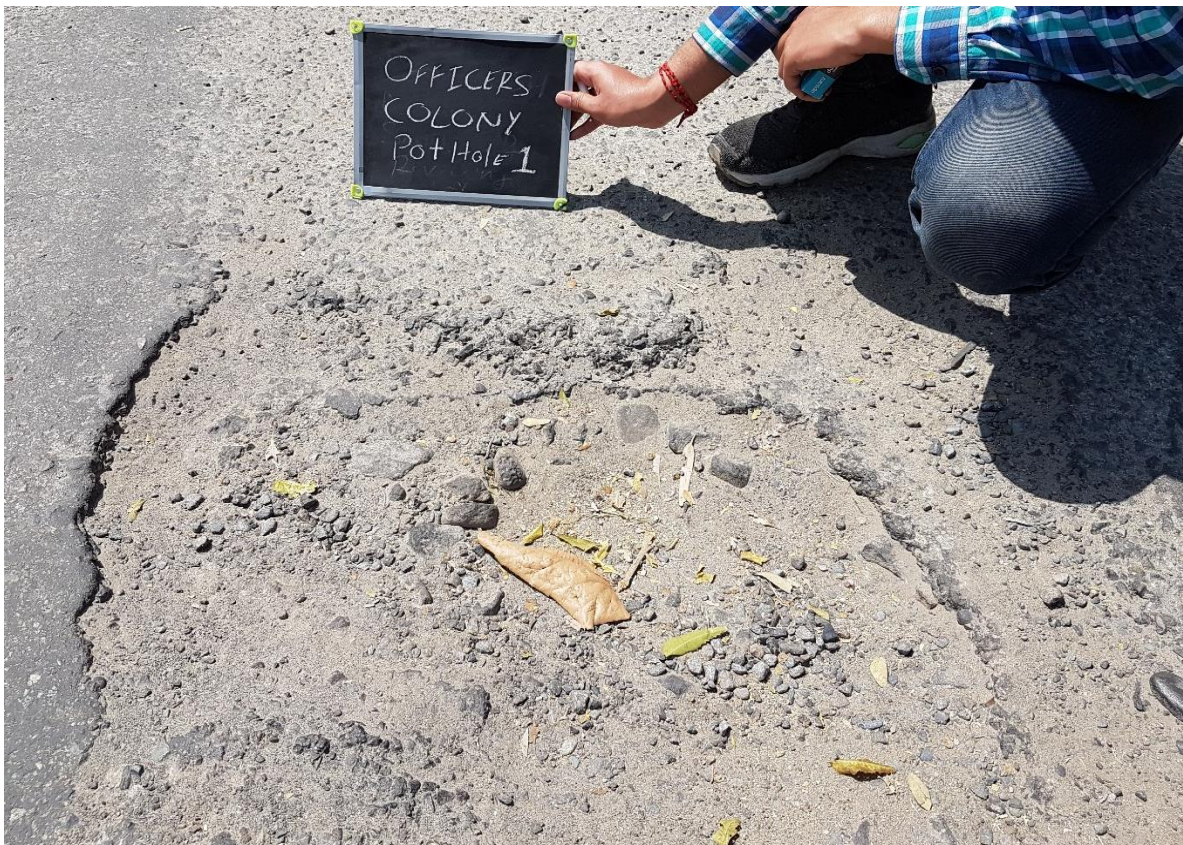
Figure 4.11: Pothole at section OC
