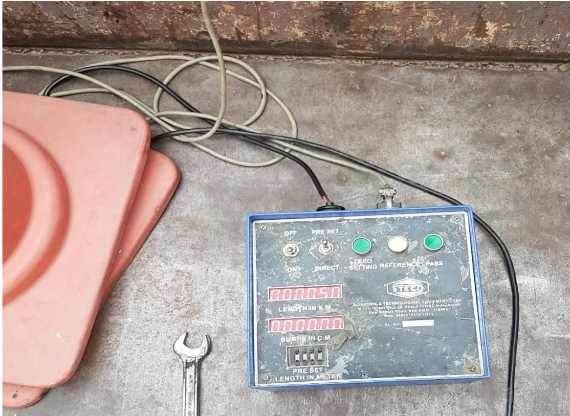
Figure 4.18: Readings Displayed on Panel Board Placed in Back of Towing Vehicle
