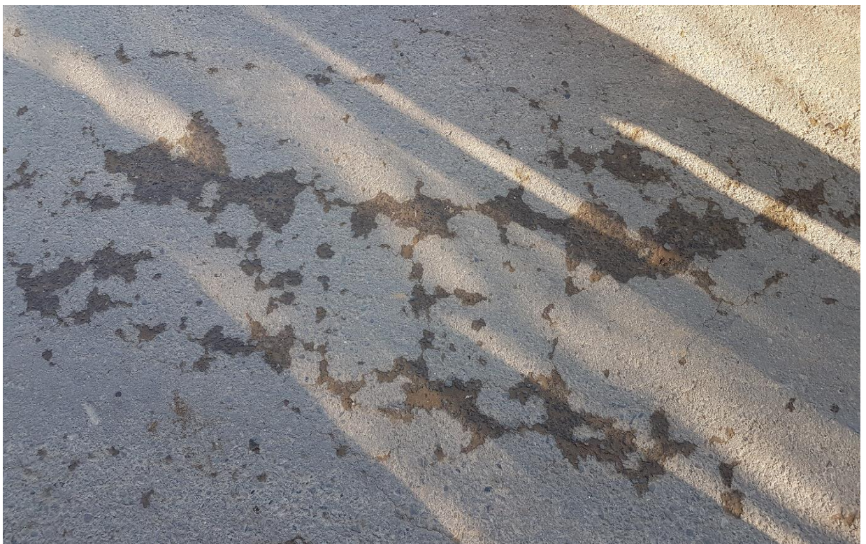
Figure 4.5: Cracking on Section AN
