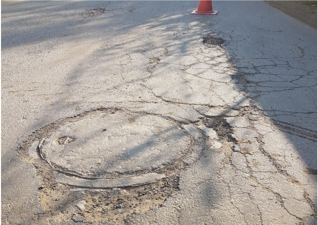
Figure 4.6: Cracking Due to Manhole Uplift
