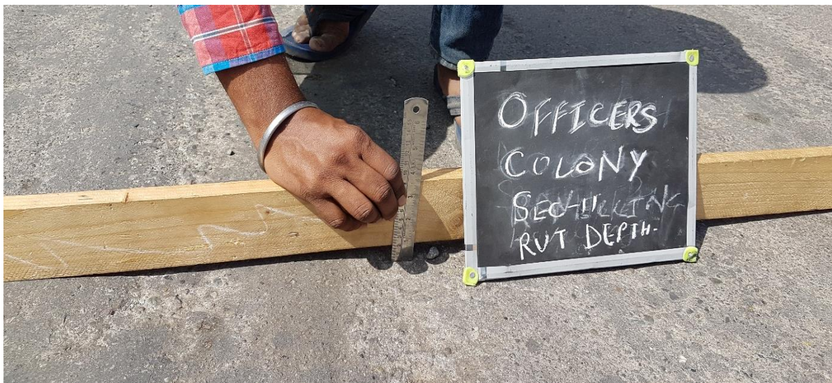
Figure 4.12: Rutting Measurement at OC Section
