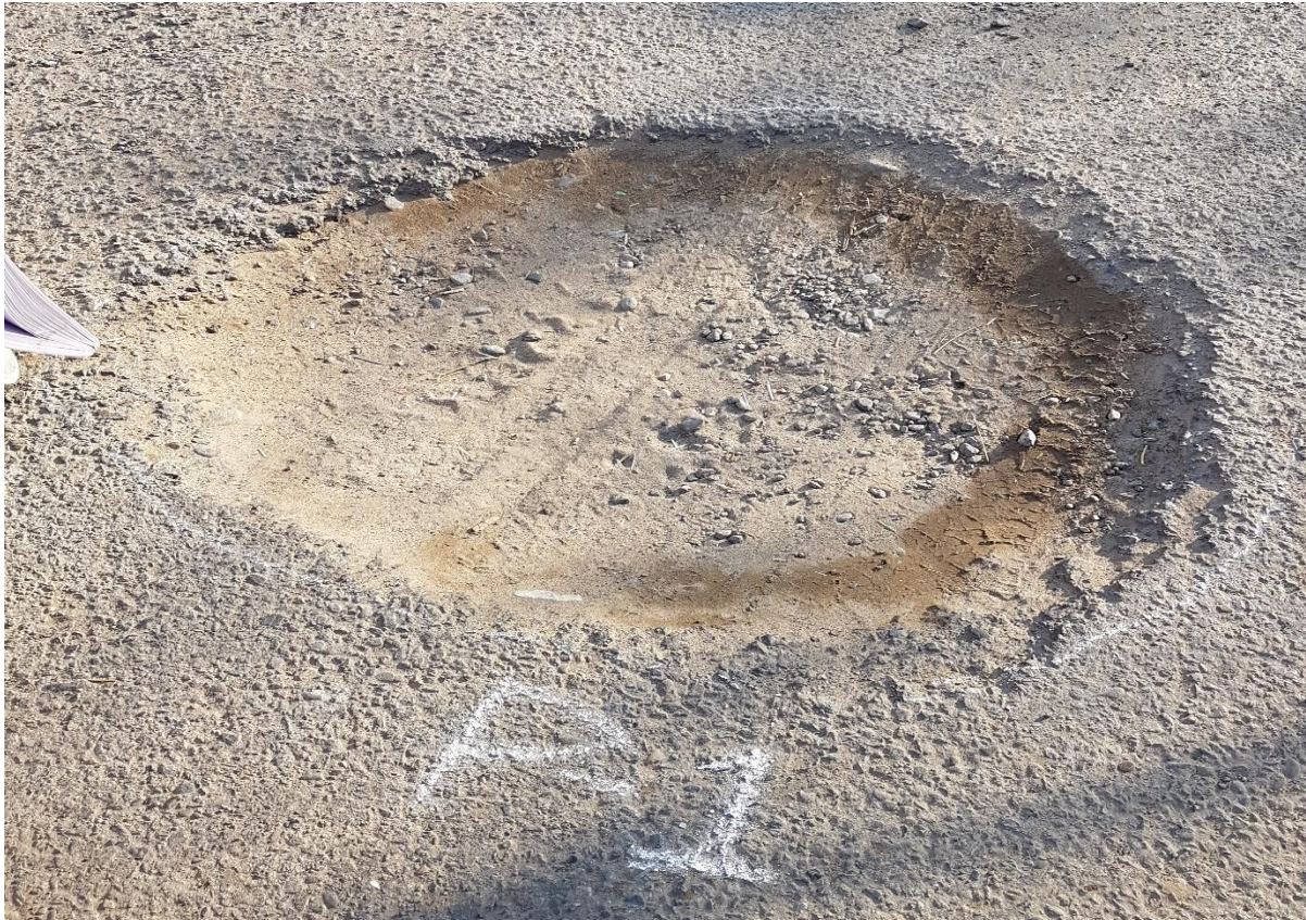
Figure 4.10: Pothole on Section PN
