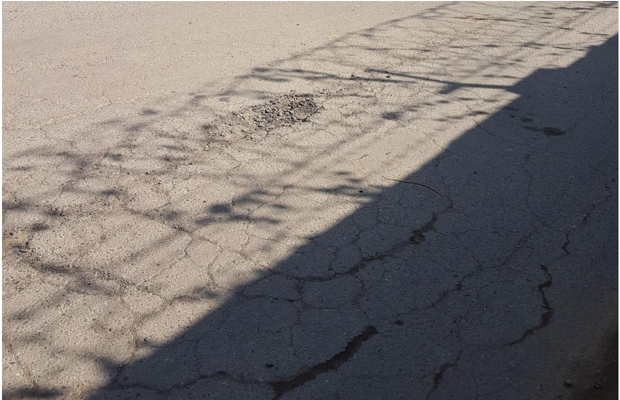
Figure 4.4 : Cracking on Section PN
