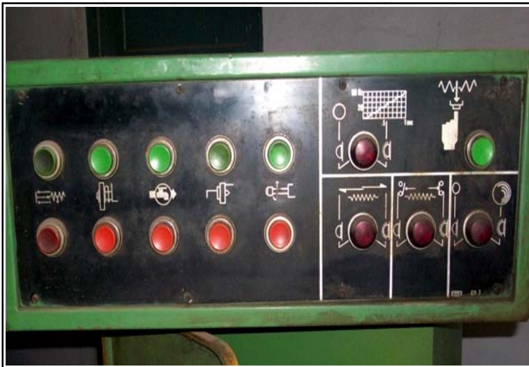
Figure 5.3: Control Box Panel
