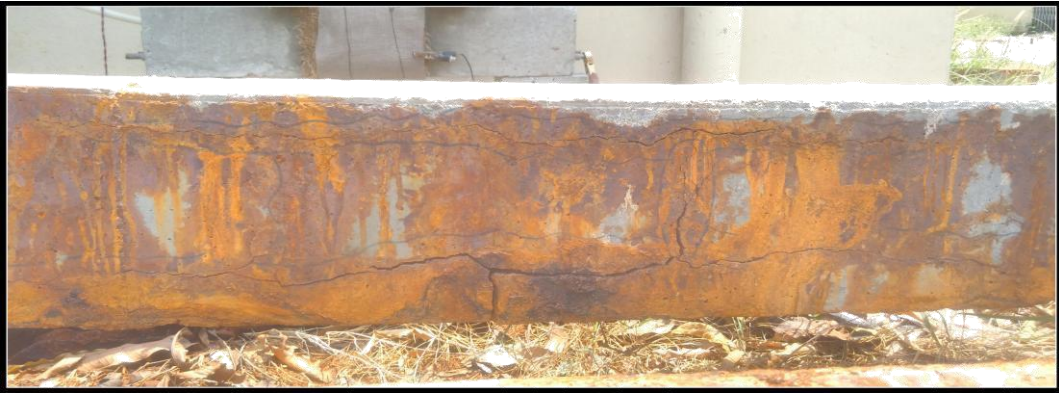
Fig 4.6 Longitudnal and tranverse cracks at right face of C-15
