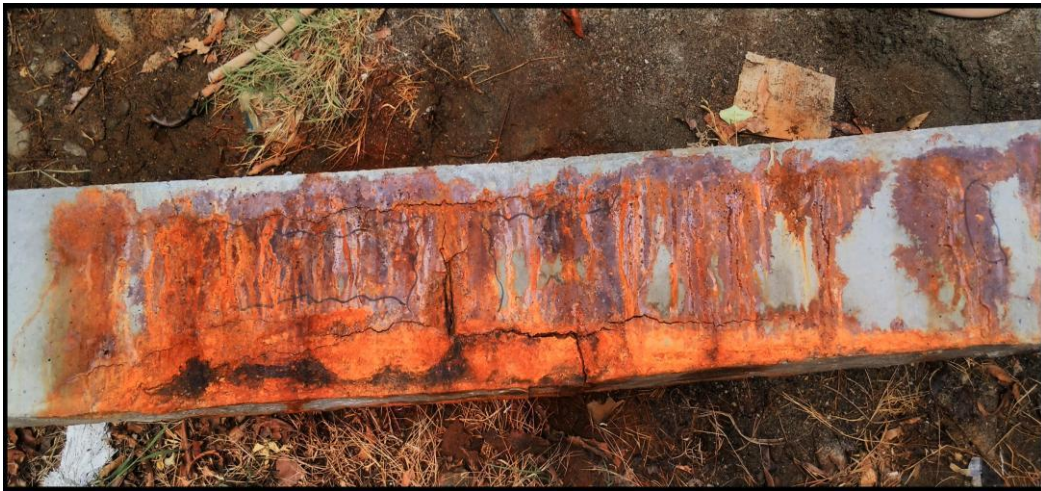
Fig 4.7 Cracks on left face of C-15
