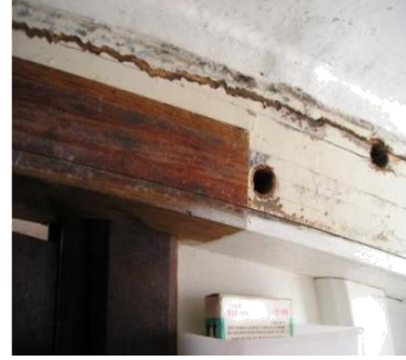
(2) Corrosion in beams
