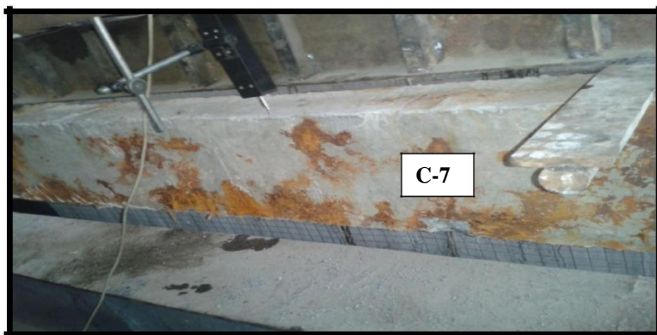
Fig 4.16 Side face of C-7 Beam before load
