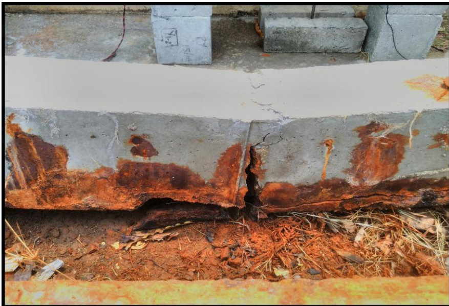
Fig 4.11 Dark reddish brown corrosion products
