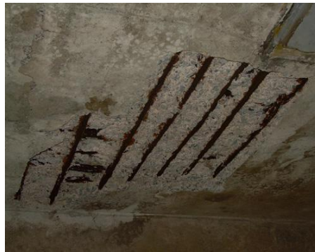
(3) Corrosion in slabs
