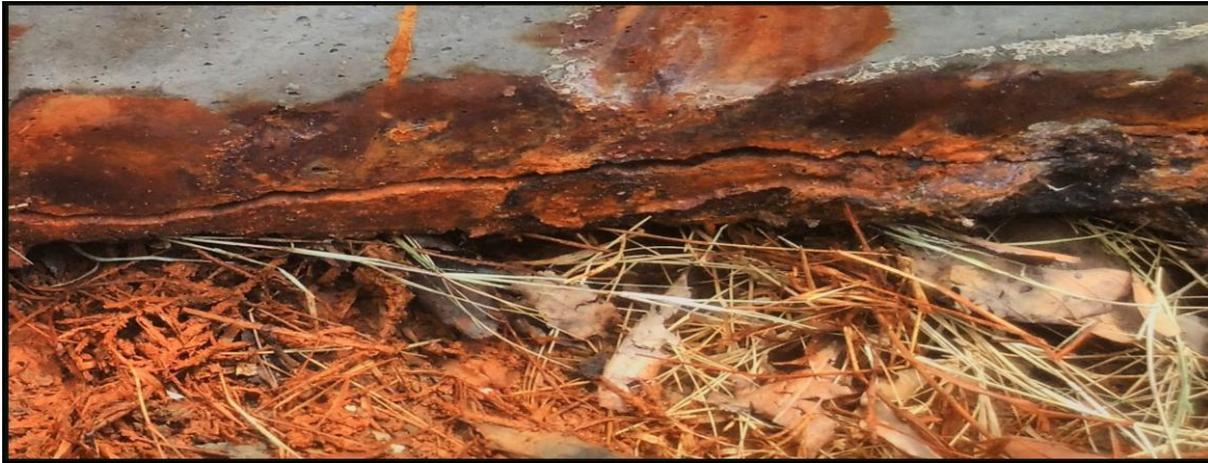
Fig 4.12 Long horizontal cracks at the bottom side of front face
