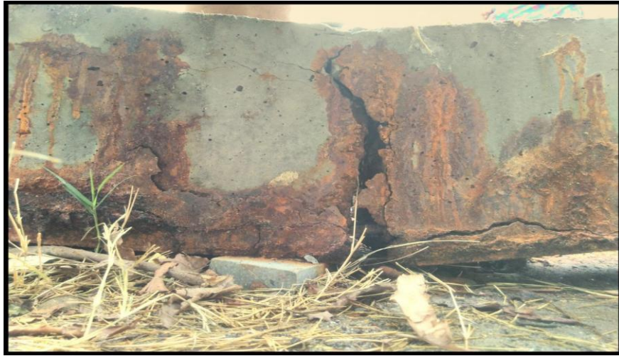
Fig 4.10 Long vertical crack at centre of beam results in breaking of beam
