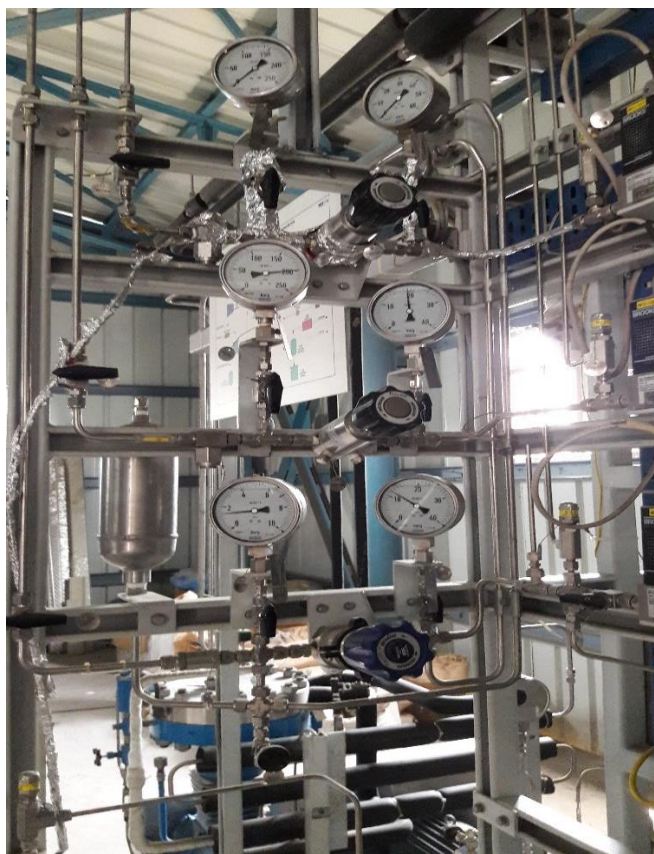
Figure 26 Inlet Section of Reformer
