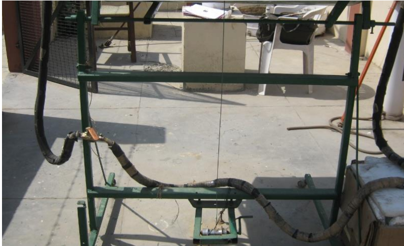
Fig.40 Insulation on pipes
