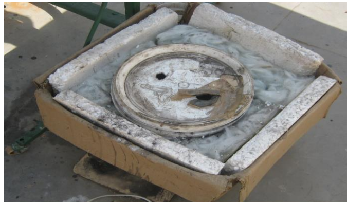
Fig.41 Insulation around the storage tank
