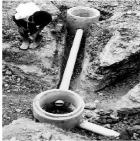
Fig: 2.3 Junction chamber in Pakistan
