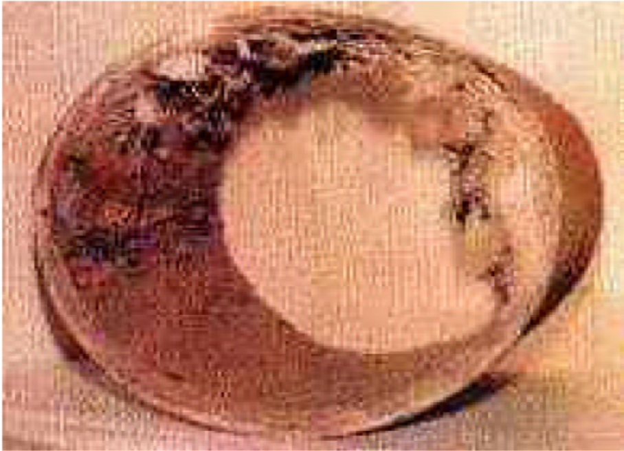
Fig: 2.7 235 mm asbestos pipe showing the effect of 14 year of acid attack
