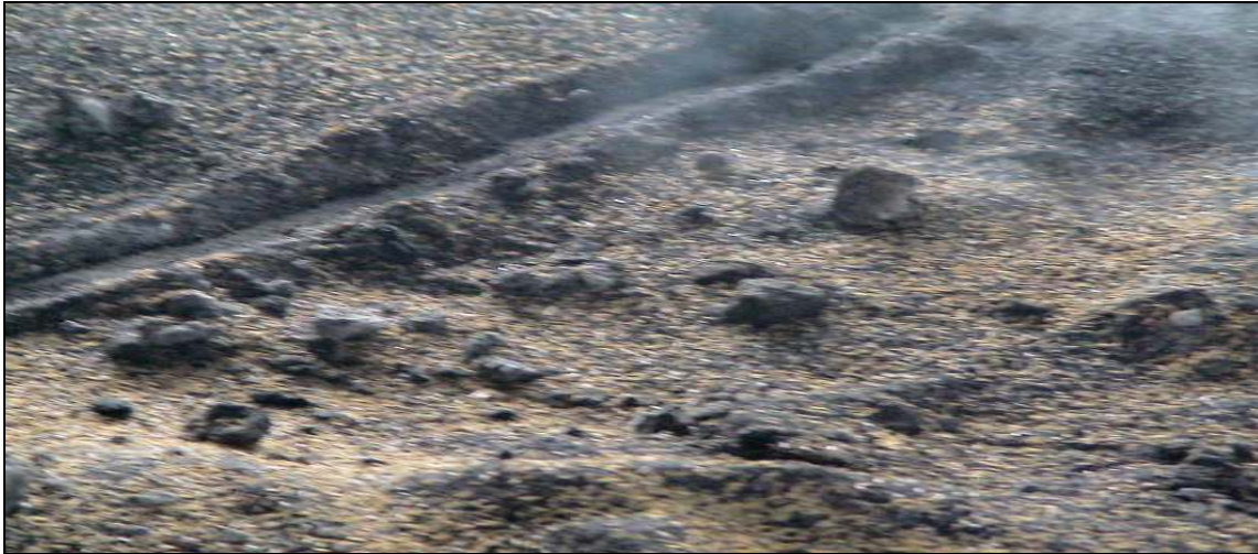
Figure 5.5 Ash agglomerates at the bottom of furnace of fluidized bed combustor at JPP
