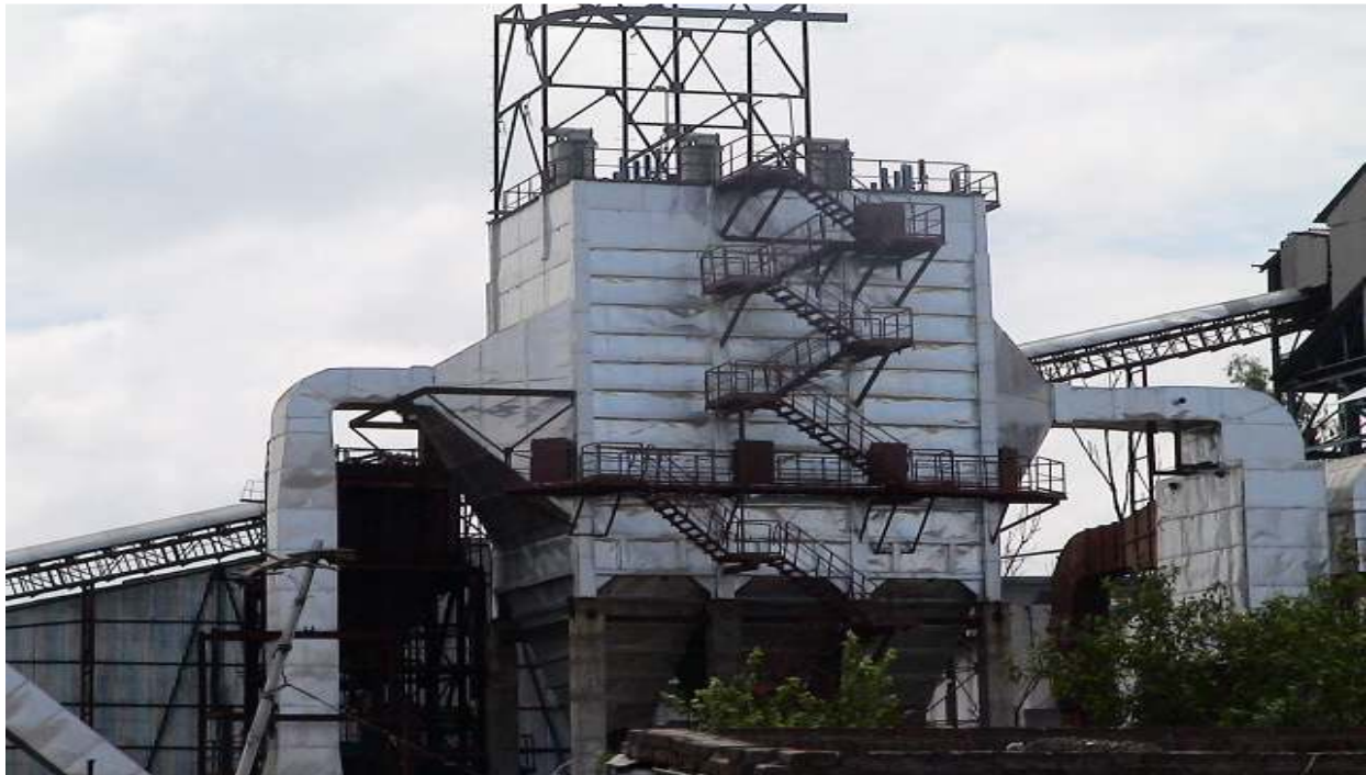
Figure 3.9 Atmospheric bubbling fluidized bed combustor at cogeneration plant at CPPDK
