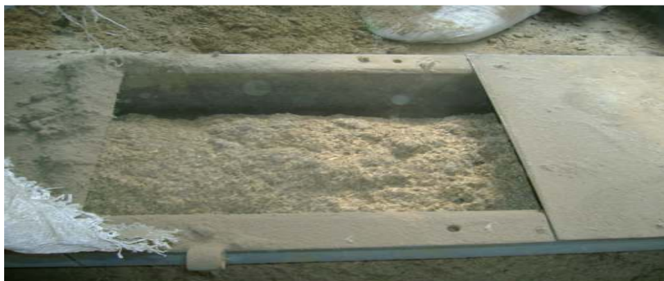
Figure 3.5 Arrangement shows the rice husk after the conveyor belt to atmospheric bubbling fluidized bed combustor at Jalkheri power plant
