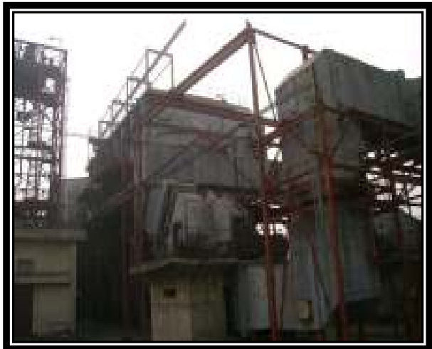
Figure 3.2 Bubbling fluidized bed combustor at JPP
