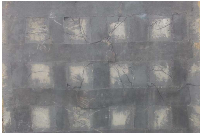
Fig. 6.9: Crack Pattern in FS 15 BFRP BD
