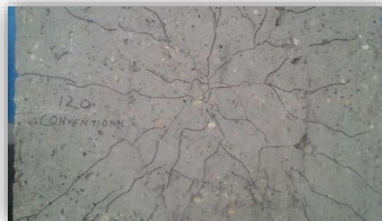
Fig. 6.6: Crack pattern in FS 12
