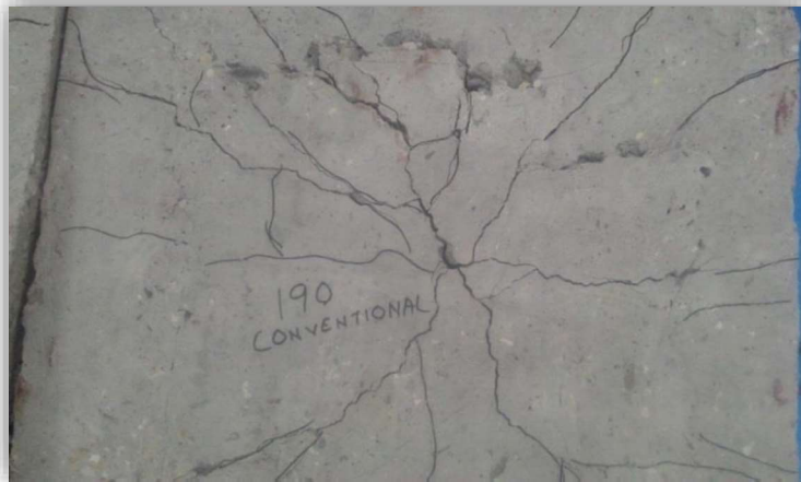
Fig. 6.8: Crack pattern in FS 19
