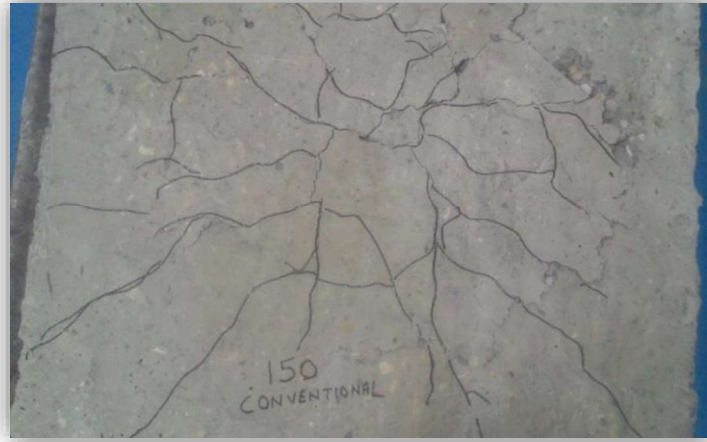
Fig. 6.7: Crack pattern in FS 15
