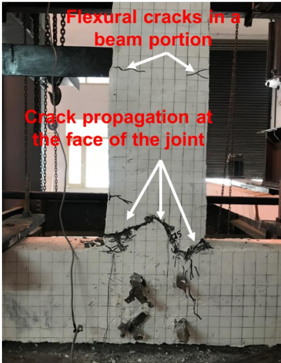
Fig. 6.33 - Crack Pattern of Wire Mesh Confined HP-HFRC Retrofitted Control Complete Damage (WC-RCD) Specimen I
