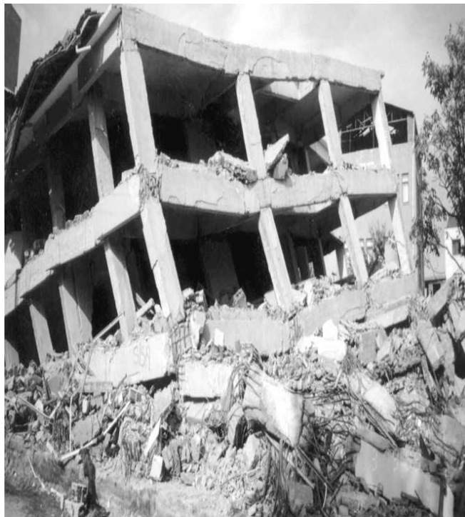
Fig. 1.6 - Shear Failure of Beam Column Joint under Strong Ground Motion in Kocaeli, 1999 ( Ghobarah and Said, 2002 )
