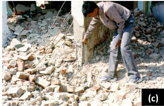
Fig. 1.1 - a) Lower Amount of Lateral Reinforcement and Poor Construction Material Led to Brittle Failure of Column Just Below the Beam-Column Junction (2001 Bhuj Earthquake); (b) Inappropriate Confinement and Maximum Lapping of Bars at One Location Led to Severe Damage and Plastic Hinge Occurred at Ground-Floor Column (2001 Bhuj Earthquake); (c) Measuring Damage Length in Ground Floor Columns ( Jaiswal et al., 2002 )
