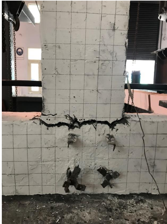
Fig. 6.45 - Crack Pattern of Wire Mesh Confined HP-HFRC Retrofitted Slight Damage (WC-RSD) Specimen I
