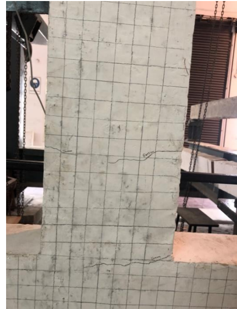
Fig. 6.16 - Crack Pattern of Control Slight Damage (CSD) Specimen II
