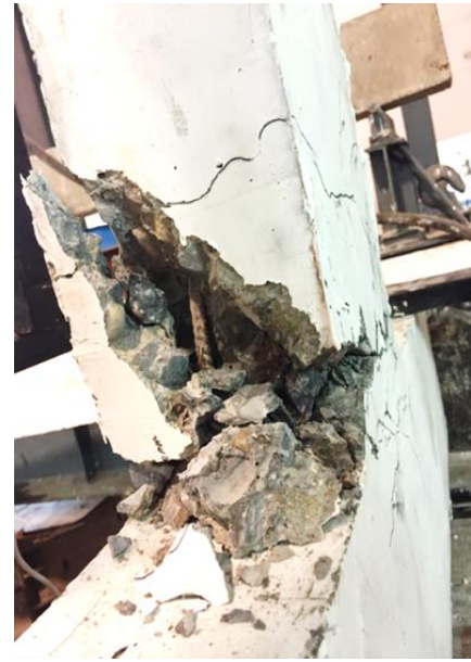
Fig. 5.3 - Crack Pattern of Control Complete Damage (C-CD) Specimen II
