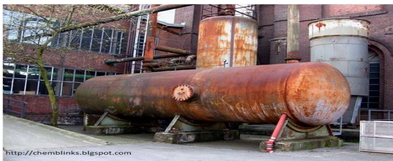
Figure 1.7 Container corroded uniformly ( http://chemblinks.blogspot.in )
