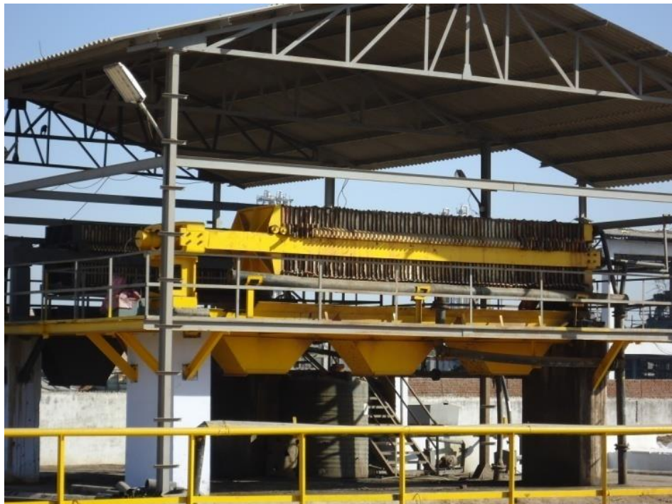
Fig. 15: Filter Press house of CETP
