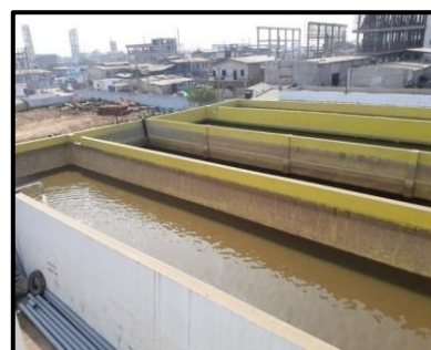
2 Equalization tanks with baffle
