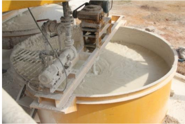
Fig. 10: Lime dosing tank of CETP
