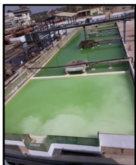
Mixing tank or Treated Effluent holding tank
