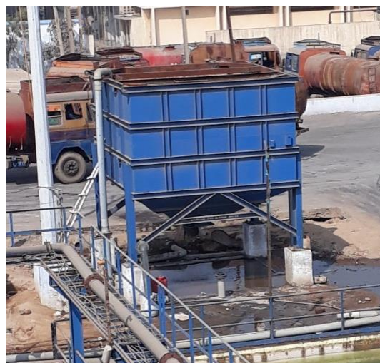
Fig. 5: Lamella Settler in CETP
