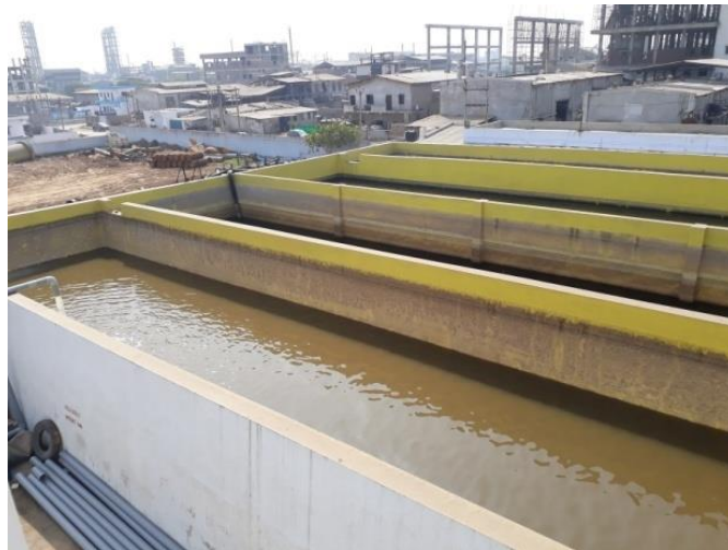
Fig. 7: 2 Equalization Tanks in CETP
