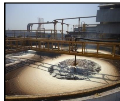
Hydrodynamic Cavitation Reactors sump
