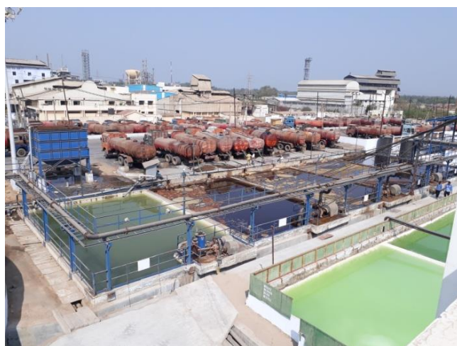
Fig. 6: 5 Collection Tanks of CETP at the back of tankers
