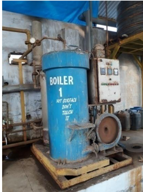
Fig. 11: Hot water boiler of CETP with small stack behind it at top.
