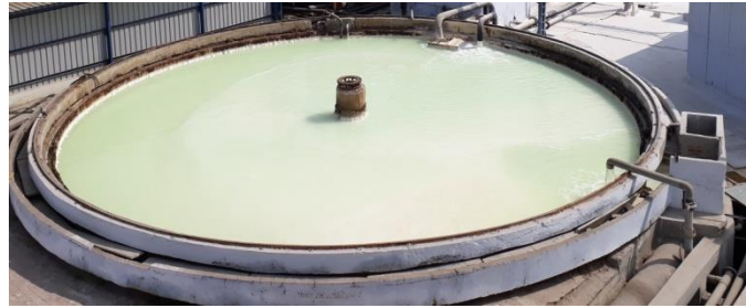
Fig. 13: Intermediate Holding Tank of CETP
