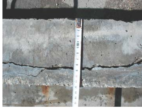
(b) Cracks on the span beam
