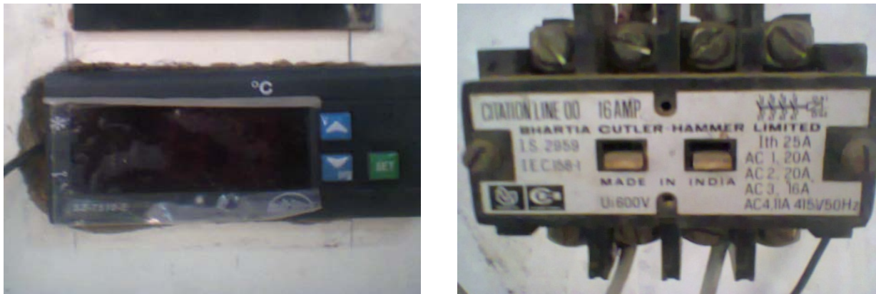
Figure 3.16 – Digital temperature controller and relay switch
