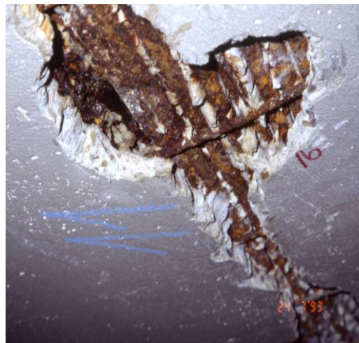
(c) Corrosion of slab
