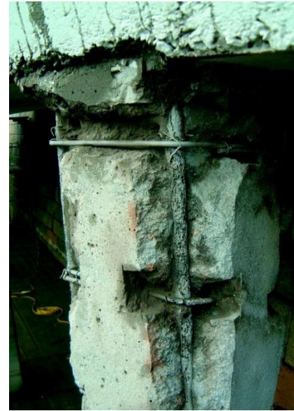
(b) Corrosion of column
