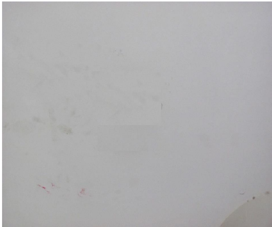
Fig. D-2. Condition of S_2 reinforced concrete slab selected for testing
