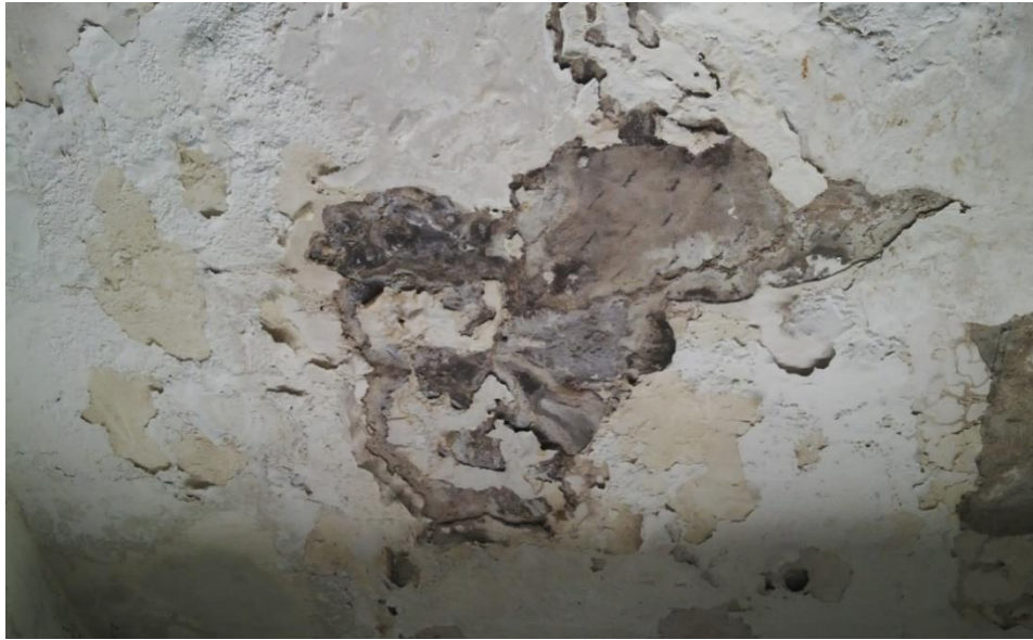
Fig. D-1. Condition of S_1 reinforced concrete slab selected for testing
