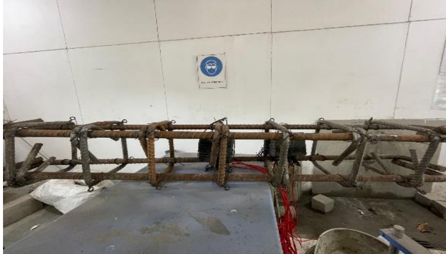
Fig3. 9 Sensor attached to the reinforcement
