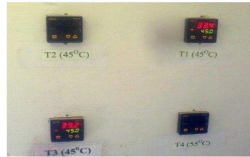
Fig. 4.15 (b) Temperature display panel with controller
