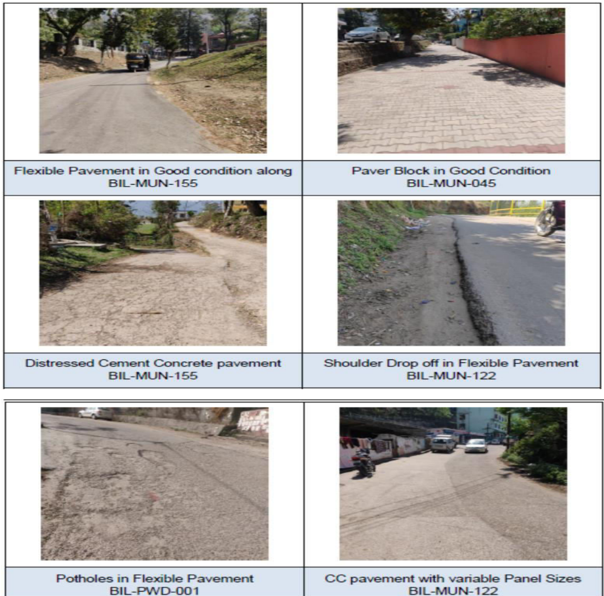
Fig.3.13: Pavement Inventory Photographs
