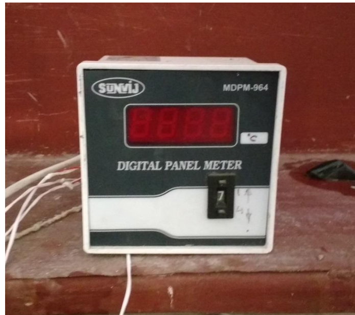
Figure 4.17: Digital panel meter
