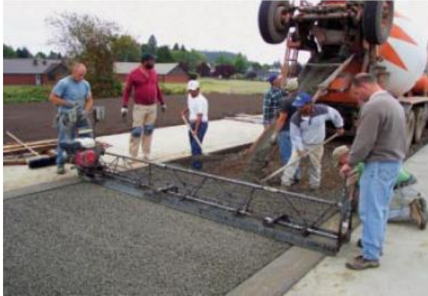
Figure 1.2: Pervious Concrete is placed and finished with a vibrating screed (Image Source: Tennis et al. 2004)
