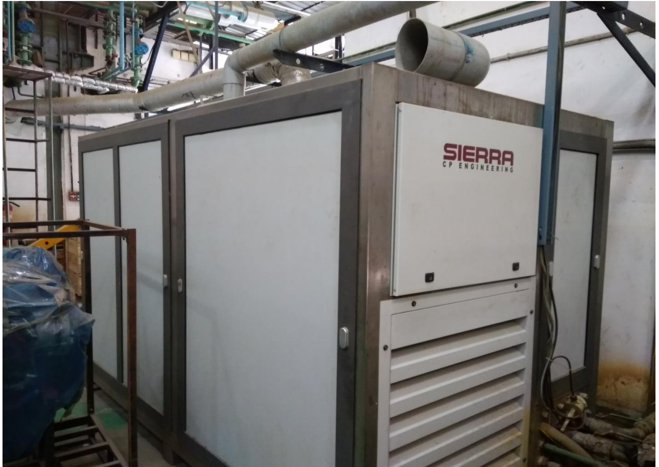
Figure 4.3 Combustion air handling unit
