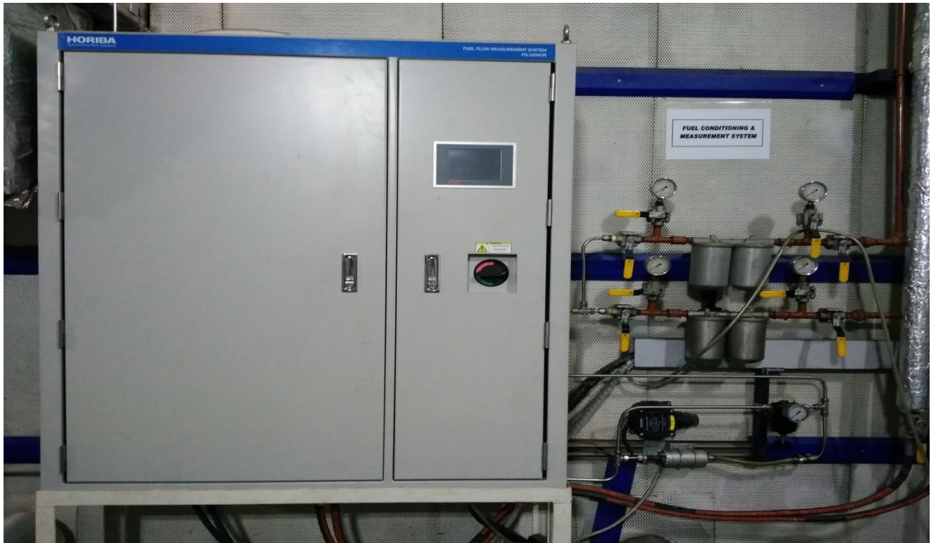
Figure 4.4 Fuel flow measuring and conditioning unit
