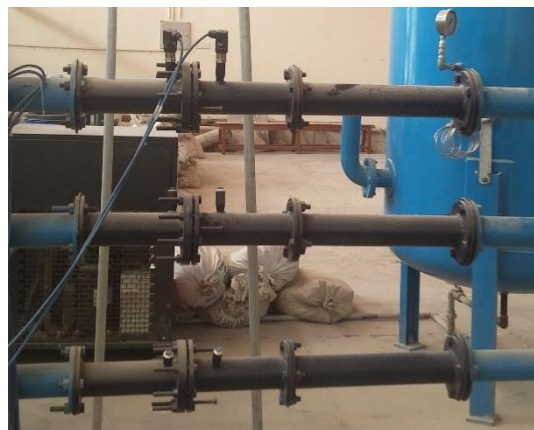
Figure 2.20 : Flowmeter in 3-inch pressure line
