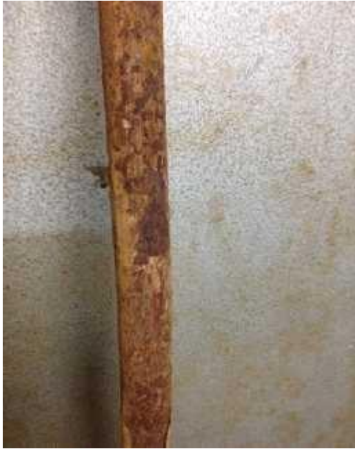
Fig.5.10 Corroded Bar of 12 mm dia
