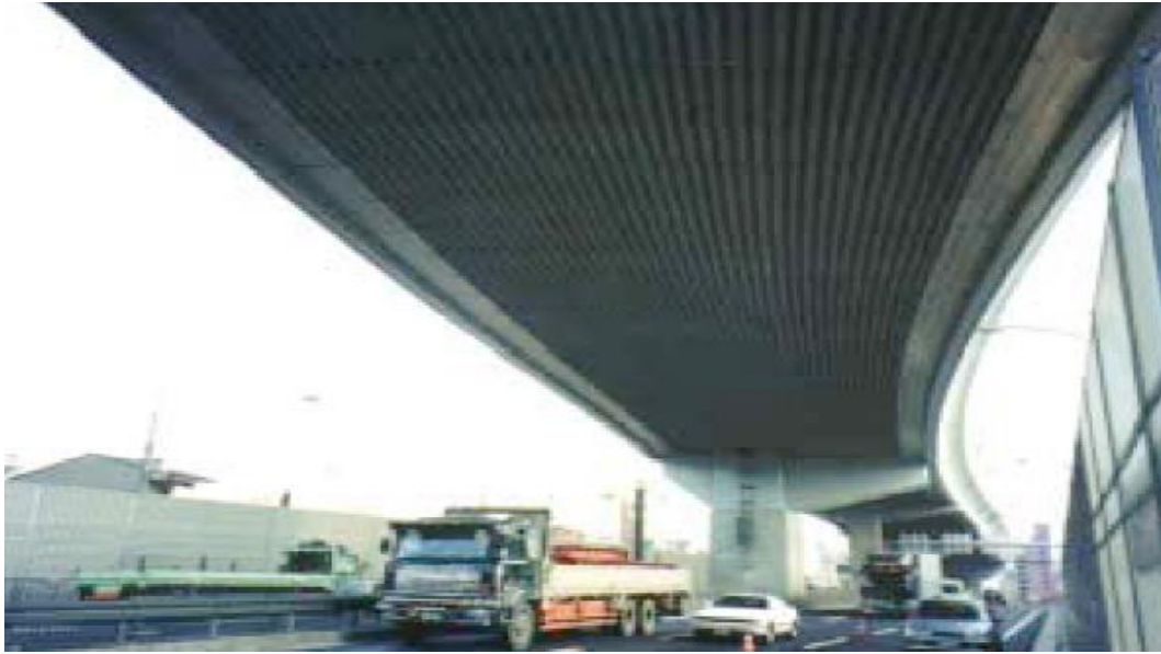
Figure 1.26: Sound absorbing structure on the under-side of an elevated via duct [Catring Kammer, 1999]
