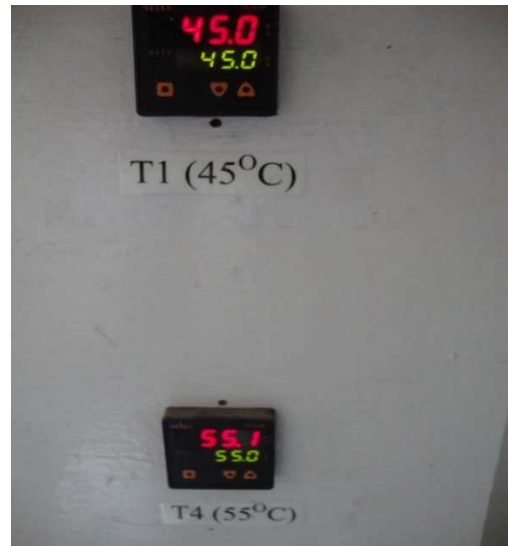
Fig. 4.7 Temperature display panel with controllers
