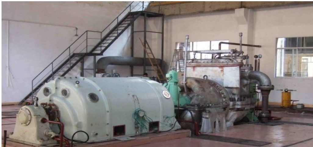
Figure3.4 steam power plant
