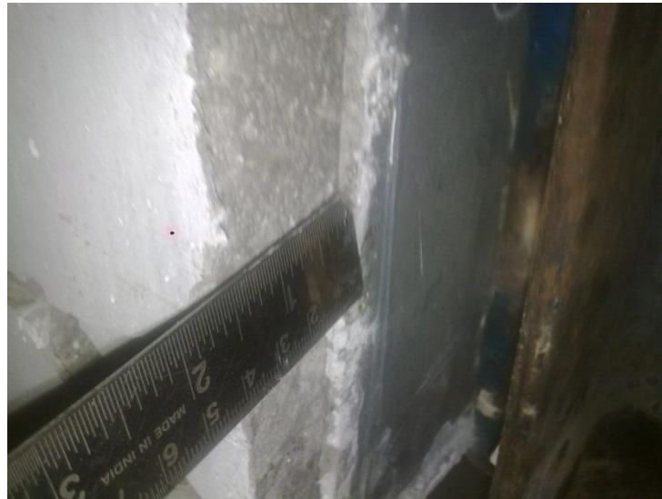
Fig 6.2 crack width in specimen 1
