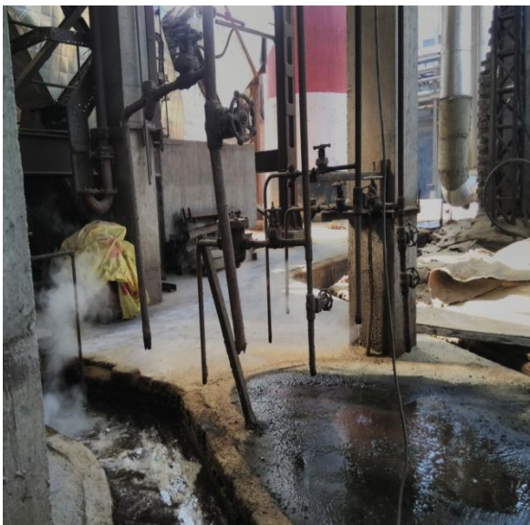
Defective Closed steam trap Near ID fan line
