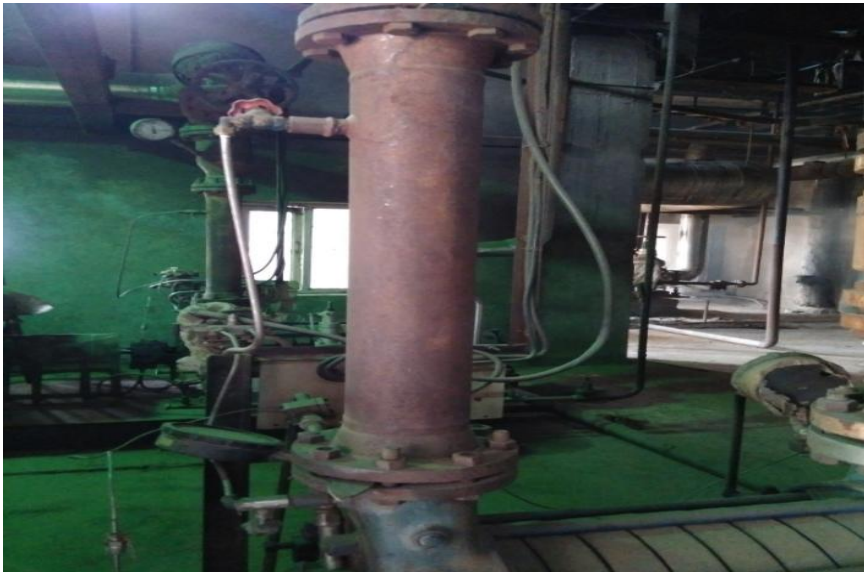
Fig- 5.5 exposed area in boiler section
