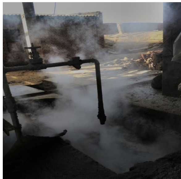
Defective open steam trap near ESP line
