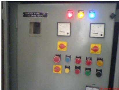
Figure 5.2 Control panel of VFD
