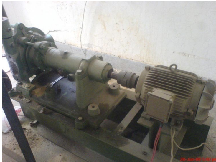
Figure 5.4 Centrifugal slurry pump of the test loop
