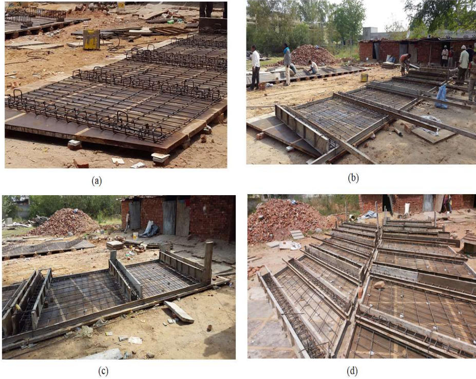
Figure 4.5: Test specimens S75B1B2B3, S60B1B2B3 and S45B1B2B3: a) Steel mesh b) After shuttering, c-d) specimen before concreting
