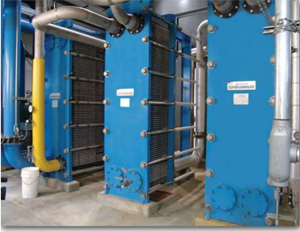
Figure 3.3: A Plate Heat Exchanger installed in industry (Source: https://www.tranter.com )
