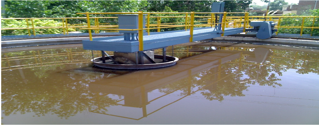
Figure 3.5: Sampling point – Secondary clarifier [P-6]
