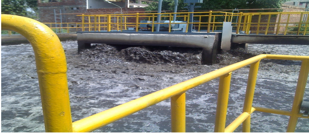
Figure 3.4: Sampling point – Parallel arrangement of two aeration tanks [Aeration tank {P-4} and Aeration tank 2 {P-5}]
