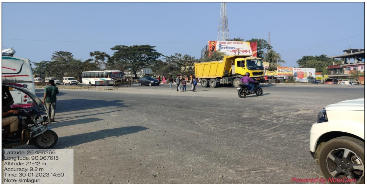
Fig 3.4 Distress, and Visible irregularities in Pavement.
