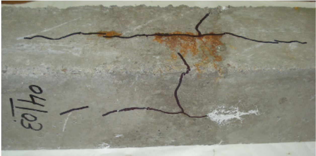
Fig.4.2: Beam showing cracks and corrosion product
