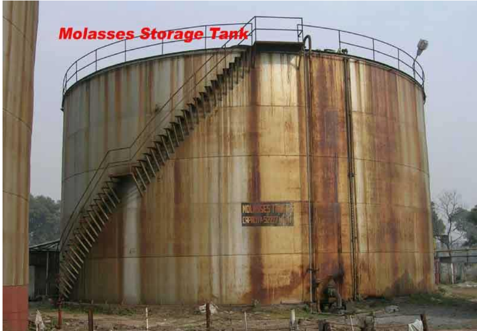
P7 – Molasses Storage Tank
