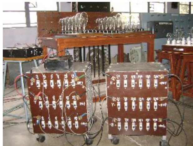
Capacitor bank and lamp load
