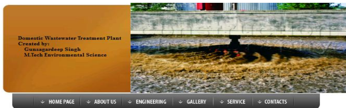
Fig 5.15 Secondary Sludge Recycle Pumps
