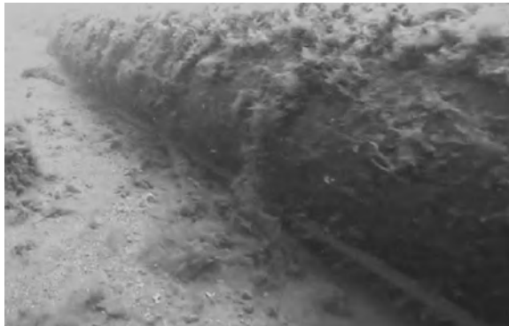
(c) Image 1 of corroded pipe
