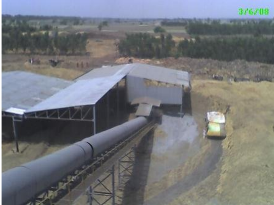
Figure 3.7: Belt Conveyor carrying fuel
