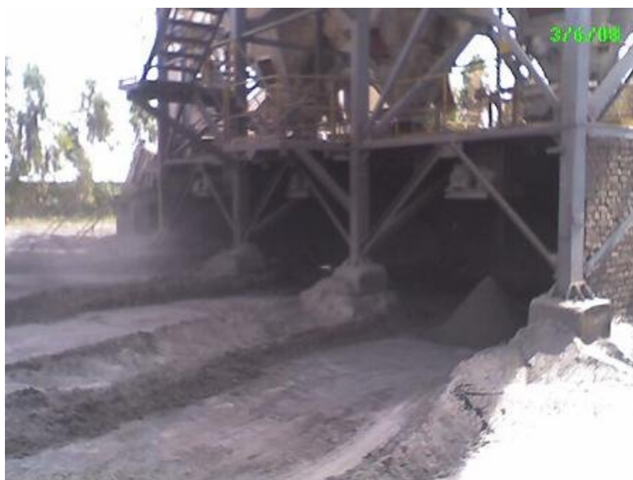
Figure 3.6: Ash under the ESP
