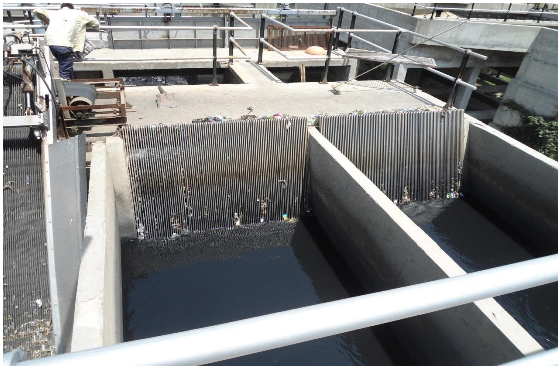
Figure 4.4: Manual screen after pumping
