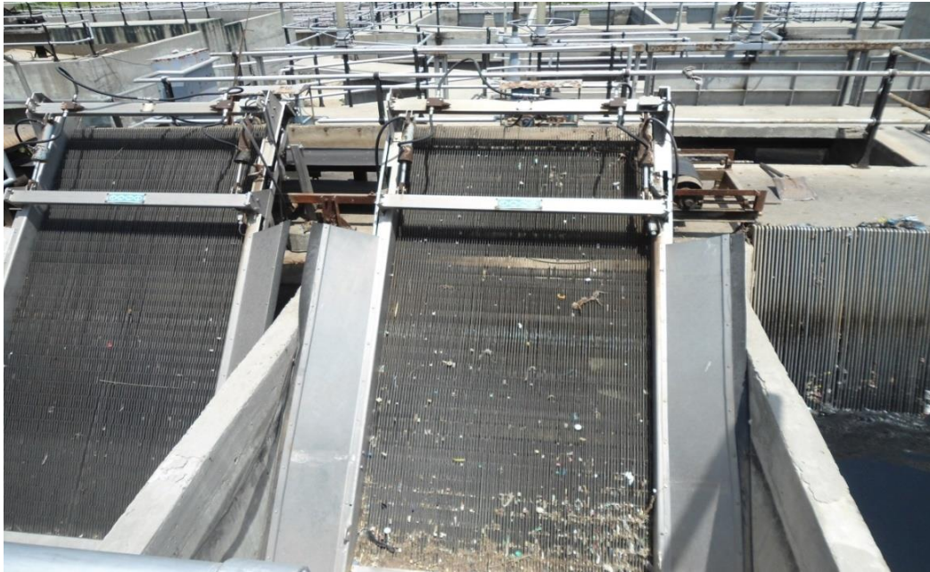
Figure 4.5: Mechanical screen after pumping
