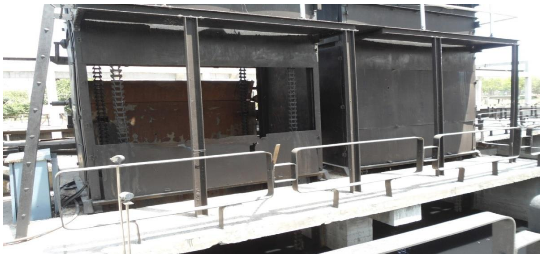
Figure 4.3: Bar screen before pumping
