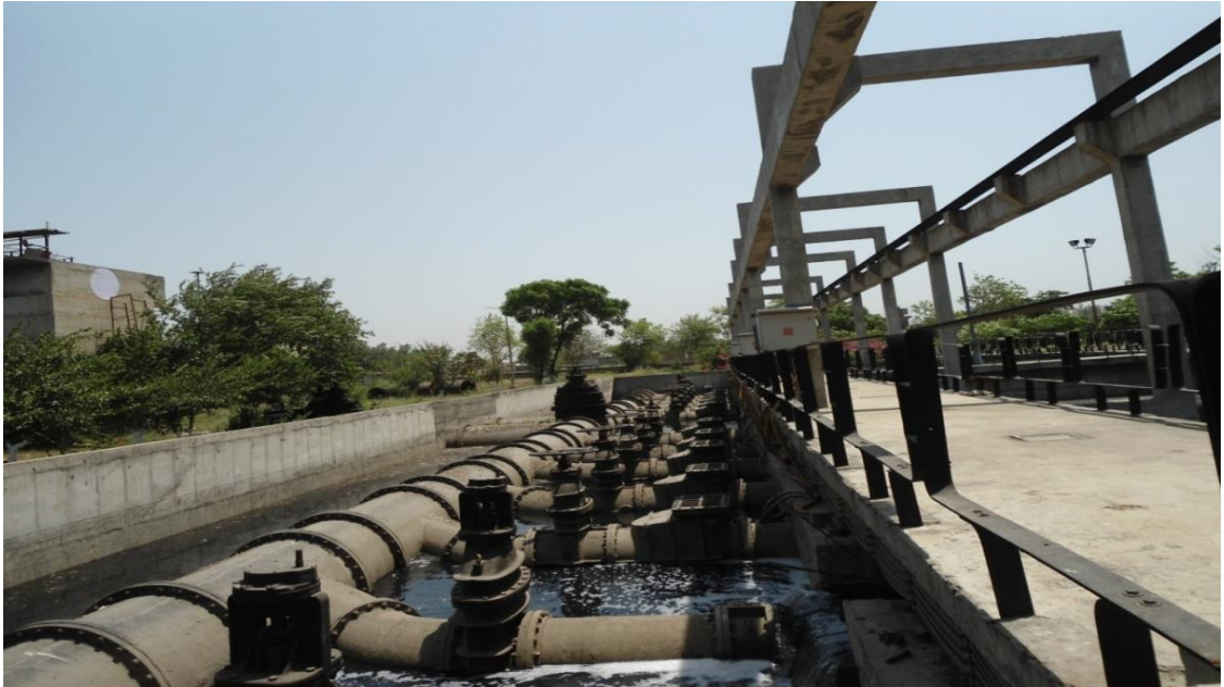
Figure 4.2: Main pumping station
