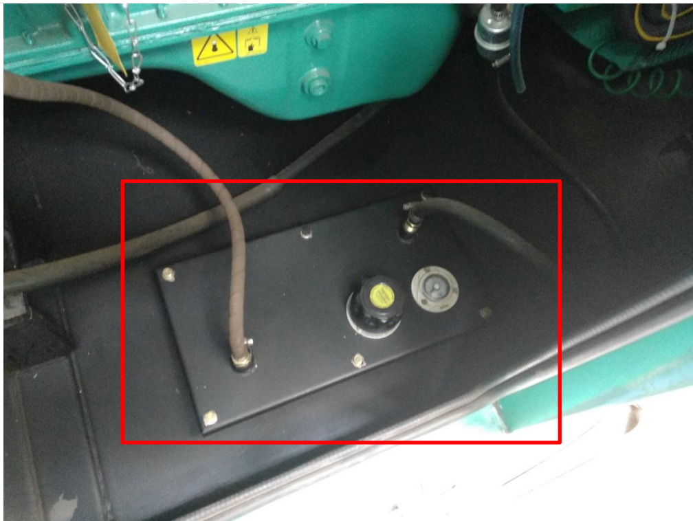
Figure 1.2 - Existing fuel filling point inside enclosure in the base rail
