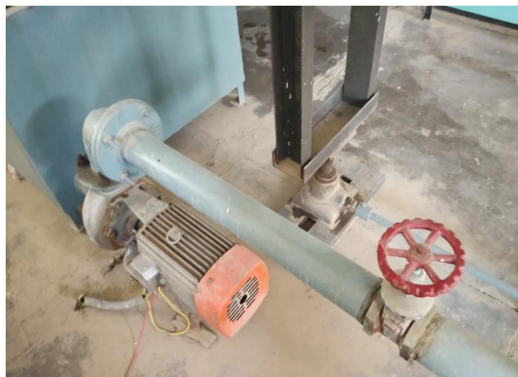
Figure 3.3 Water supply motor
