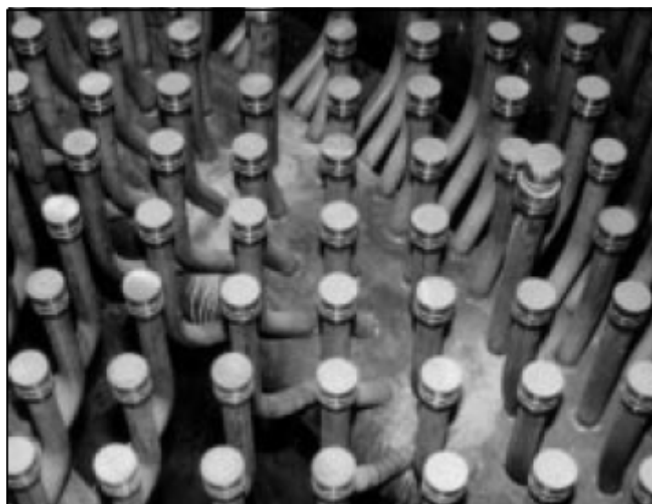
Figure 1.5 – Air pipes and bubble caps
