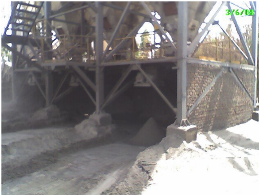
Figure 3.6 – Bottom ash under ESP
