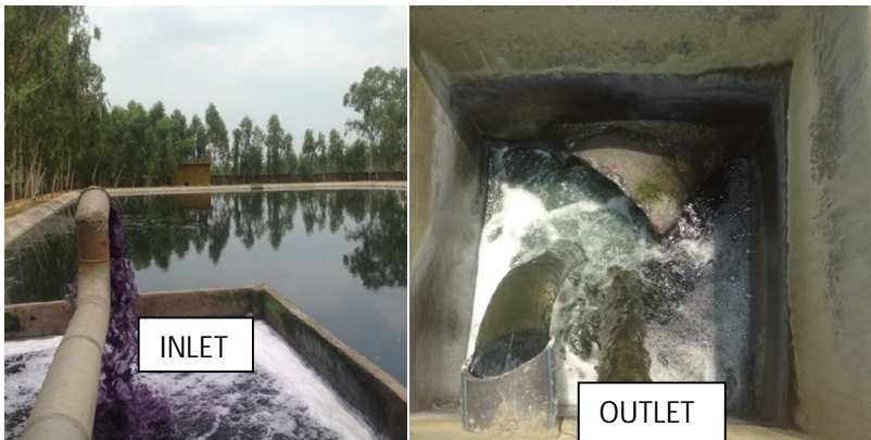
Fig 3.2 Inlet and Outlet of Anaerobic pond
