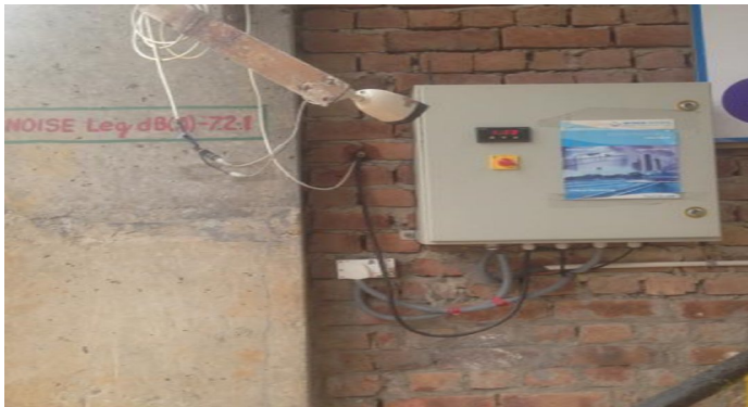
Fig 3.13 Online Monitoring System in ETP outlet
