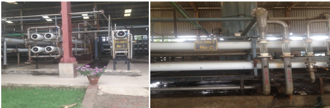
Fig. 3.11 Reverse Osmosis Units
