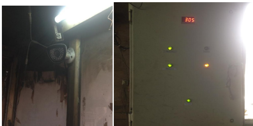
Fig 3.14 Online monitoring system for measurement of SPM in boiler stack
