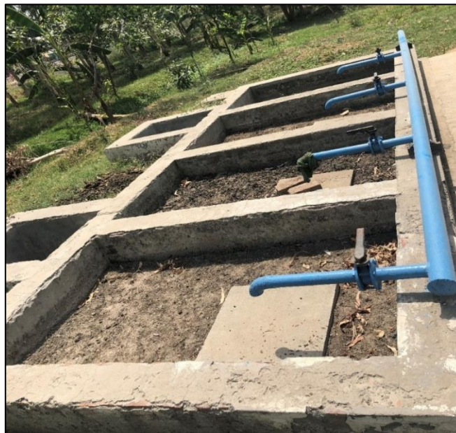
Figure 3-24 sludge drying beds
