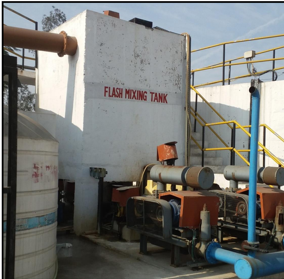
Figure 3-5 Flash mixing tank
