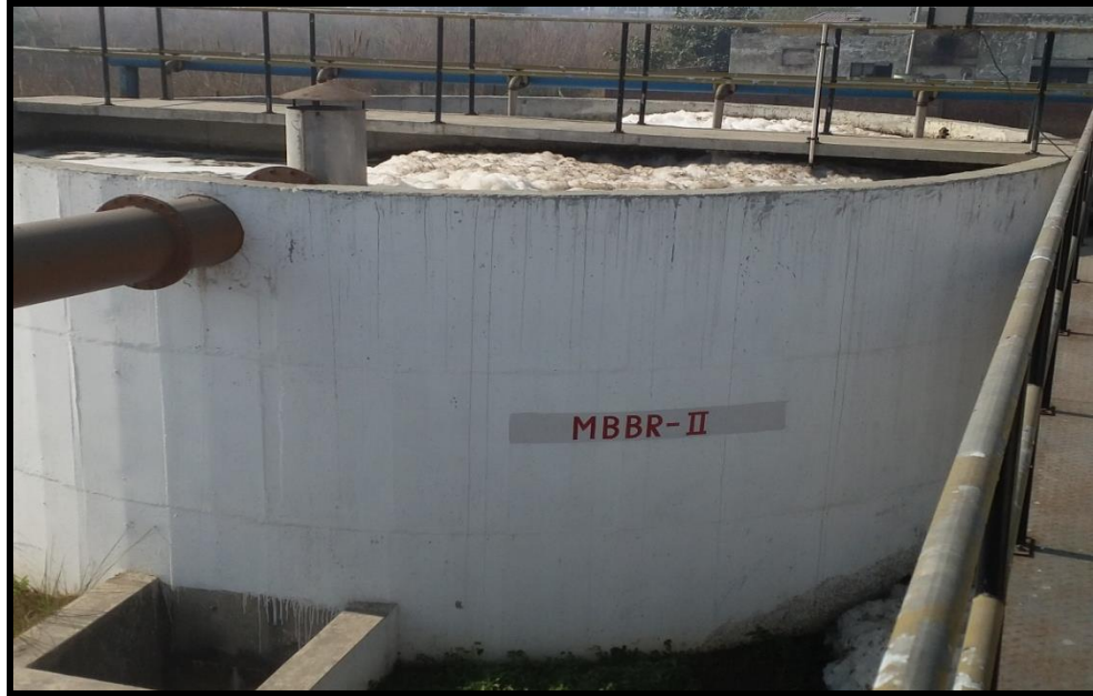
Figure 3-8 Side view of MBBR reactor
