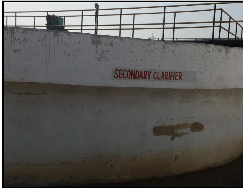
Figure 3-10 Side view of Secondary clarifier
