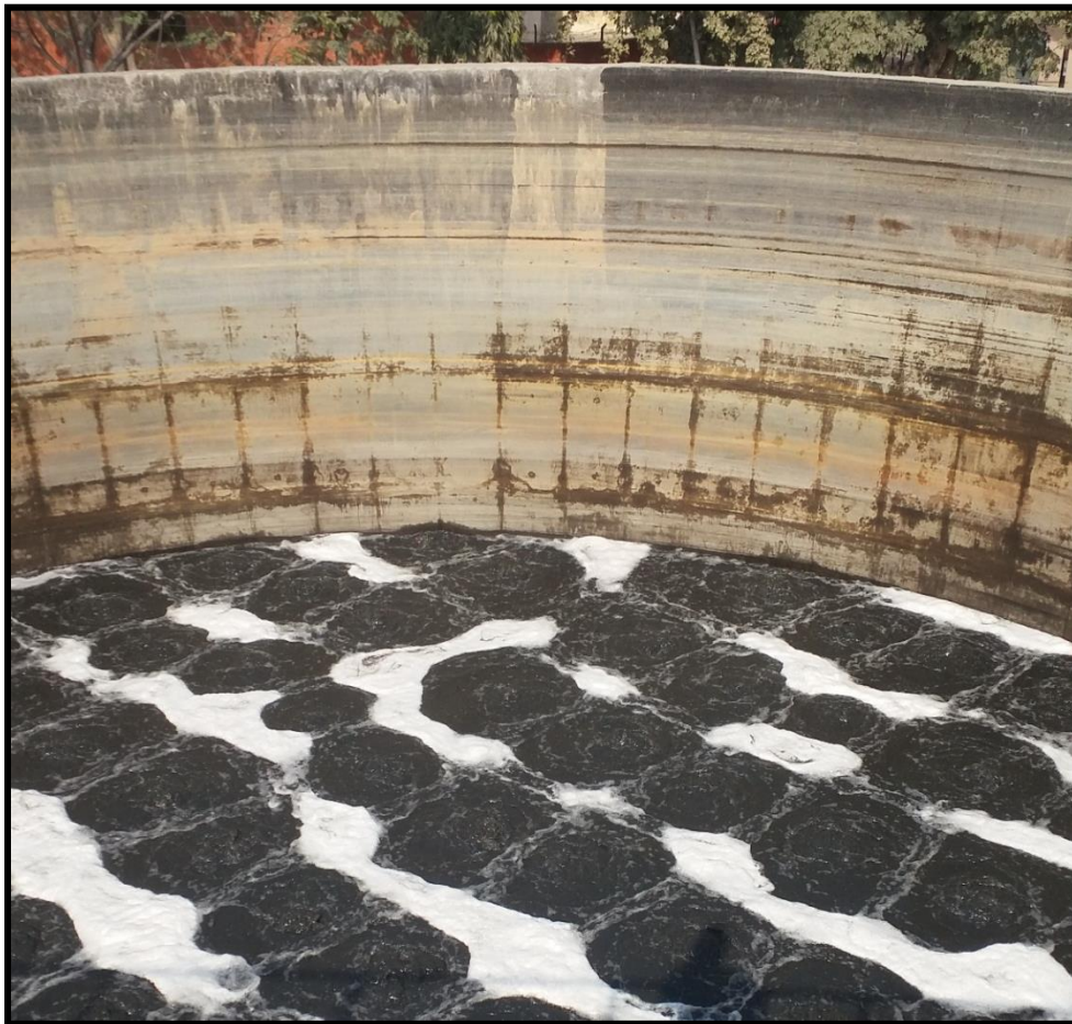
Figure 3-4 Top view of equalization tank with initial aeration process
