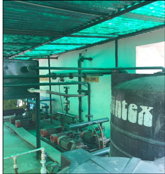
Figure 3-21 Side view of MBR tank
