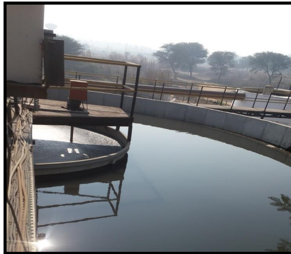
Figure 3-7 Top view of Clariflocculator
