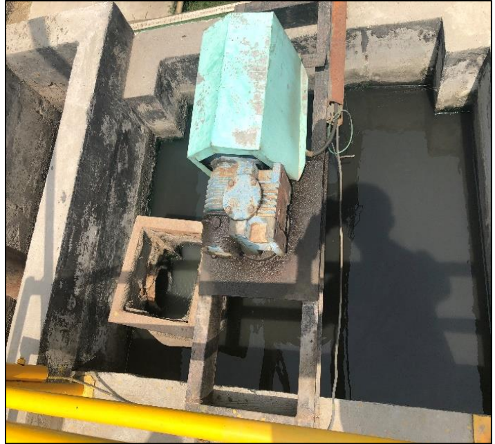
Figure 3-18 Top View of anoxic tank
