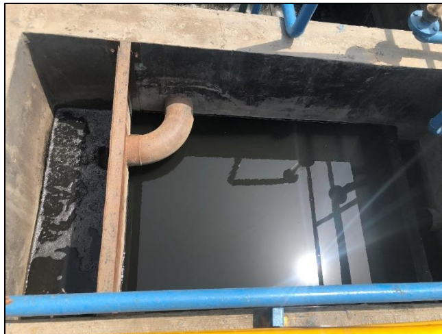
Figure 3-22 Top view of Sludge separation Tank
