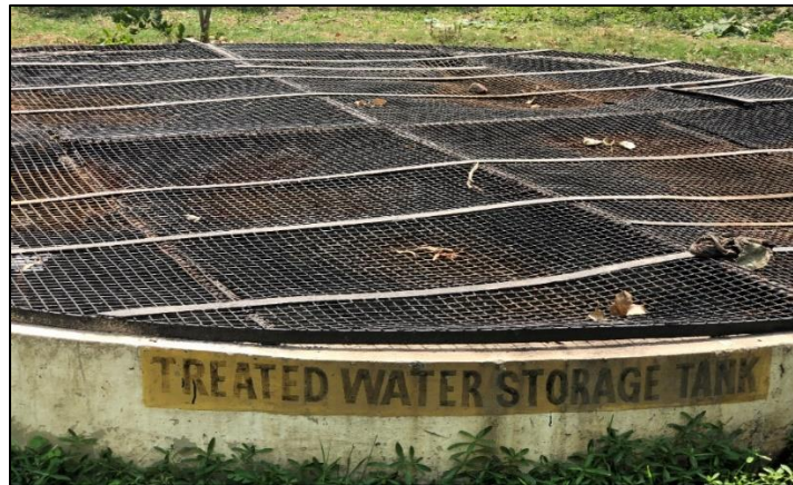
Figure 3-23 treated water storage tank
