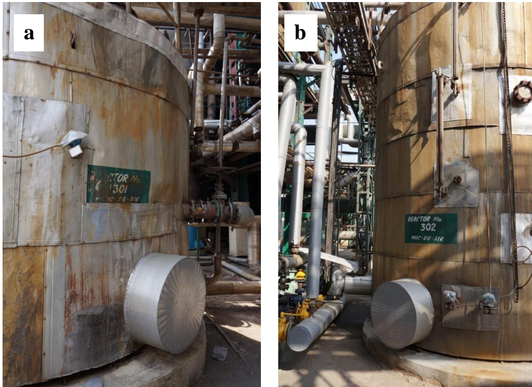
Fig. 4.2 Reactor R1 (a) and reactor R2 (b) of industrial reactor system 1
