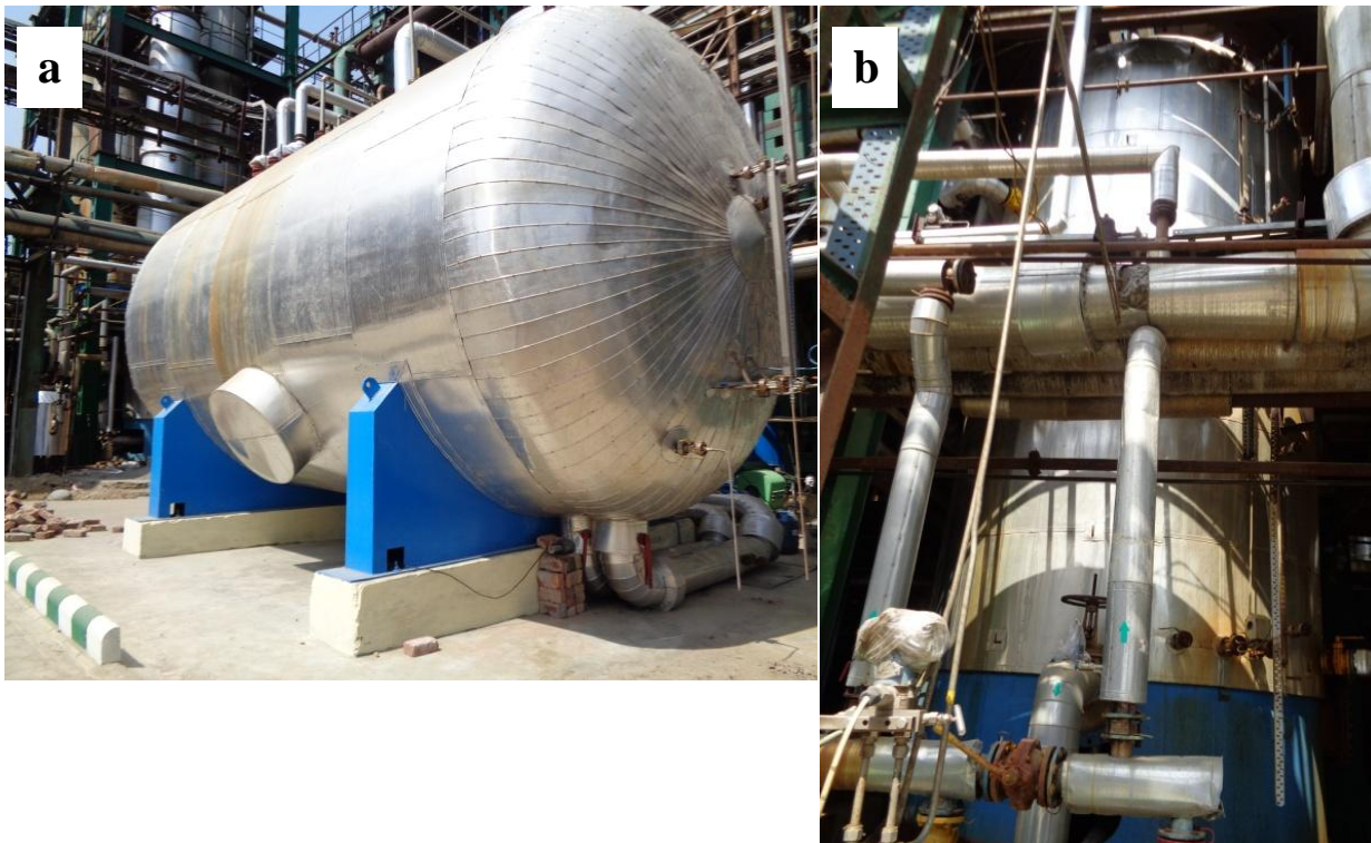
Fig. 5.2 Reactor R1 (a) and reactor R2 (b) of industrial reactor system 2
