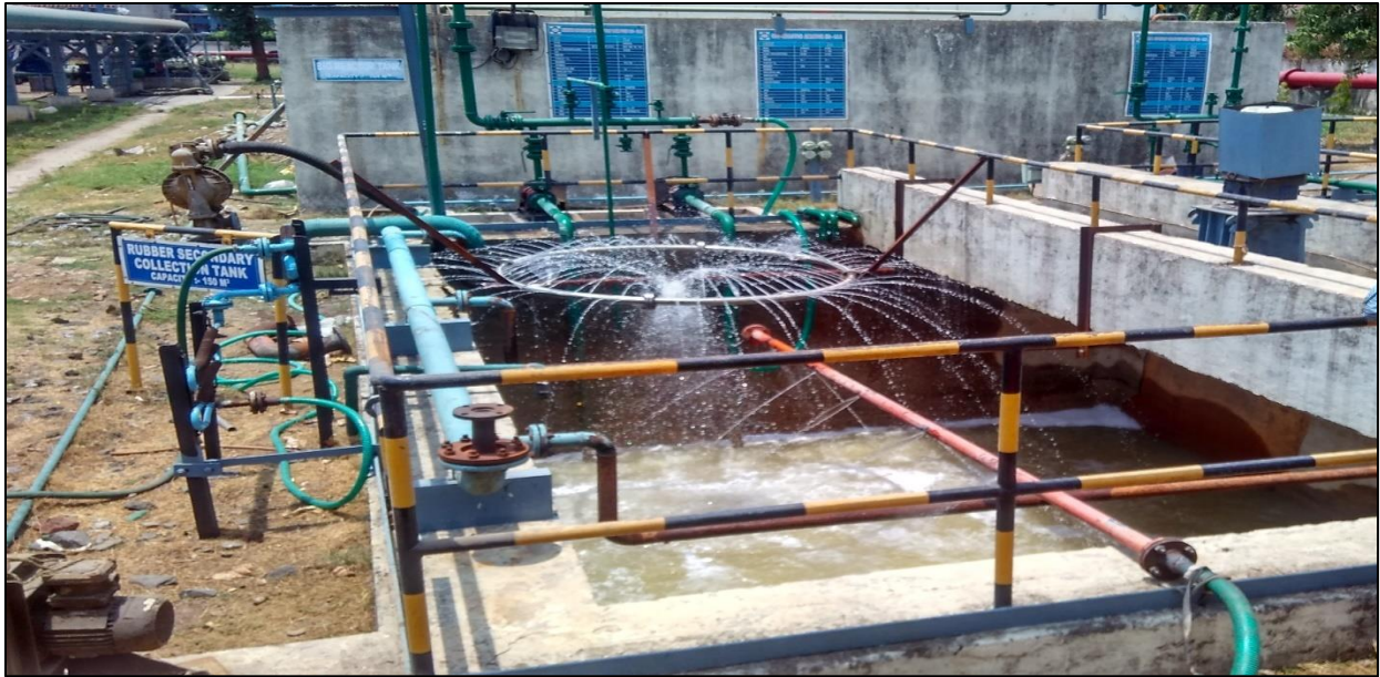
Fig. 2.7: Secondary collection tank of rubber effluent
