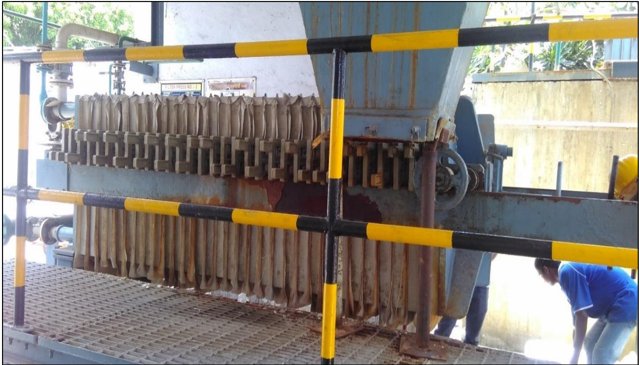
Fig. 2.10: Filter press for sludge de-watering
