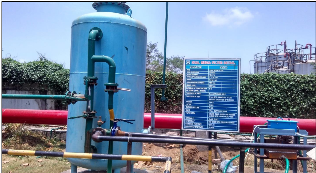
Fig 2.11: Dual media filter before final disposal to CETP
