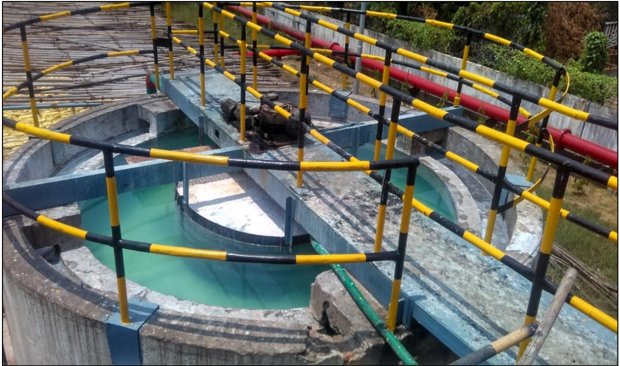
Fig. 2.5: Clarifier for latex effluent
