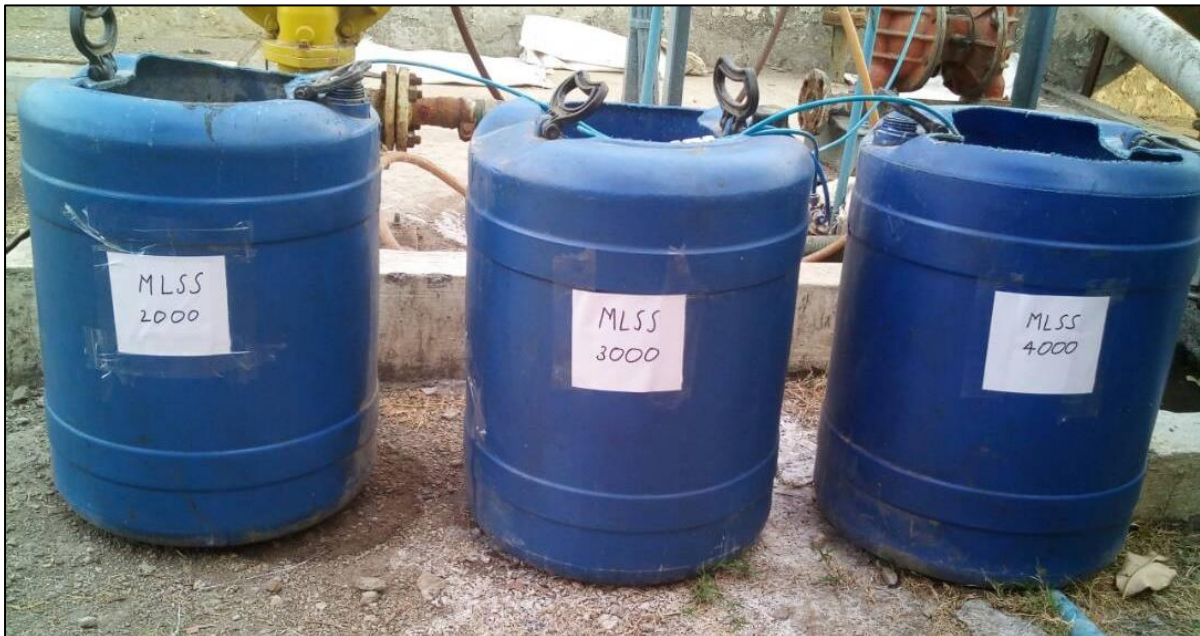
Fig. 3.9: Pilot scale bio-reactors with compressed air line
