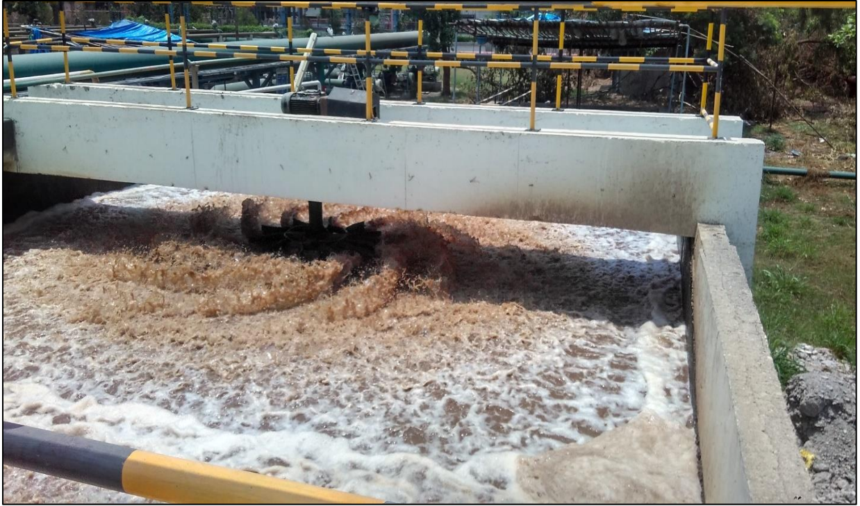
Fig. 2.8: Bio-reactor tank with surface aerator
