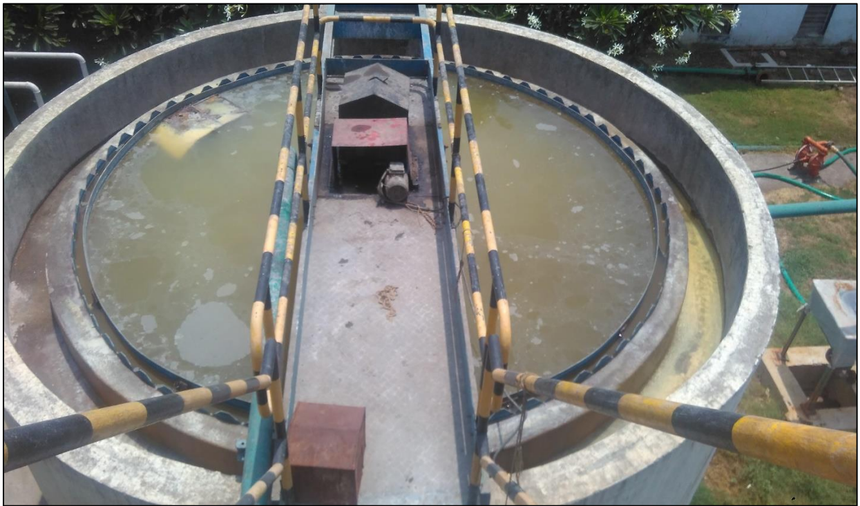
Fig. 2.6: Clarifier for rubber effluent
