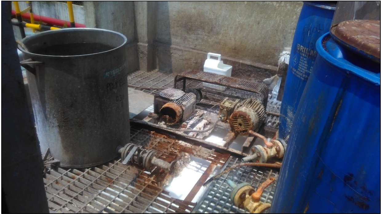
Fig. 2.4: Chemical mixing tank (Flash mixer) for latex effluent
