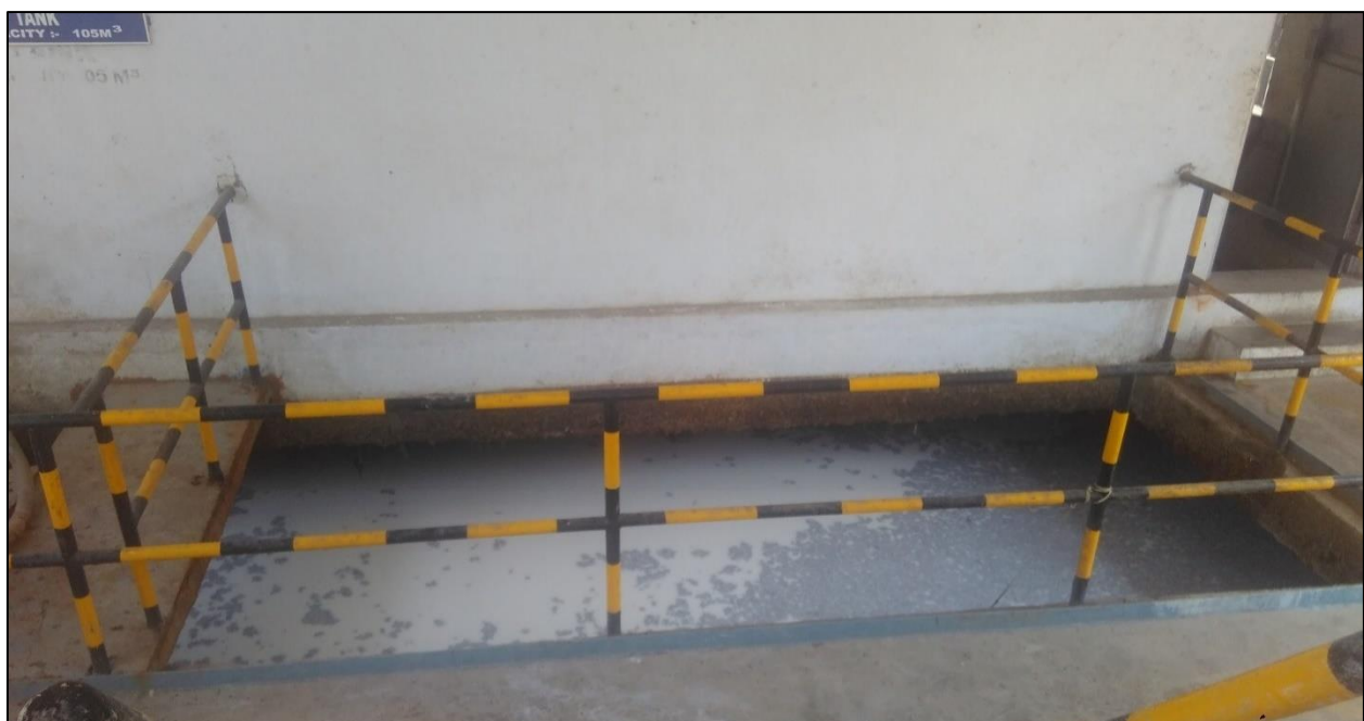
Fig. 2.3: Equalization tank of Latex effluent
