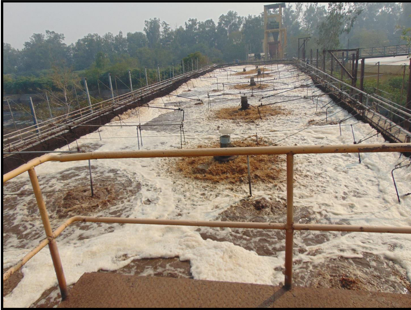
Figure 3.2 Industrial scale aeration tank-1
