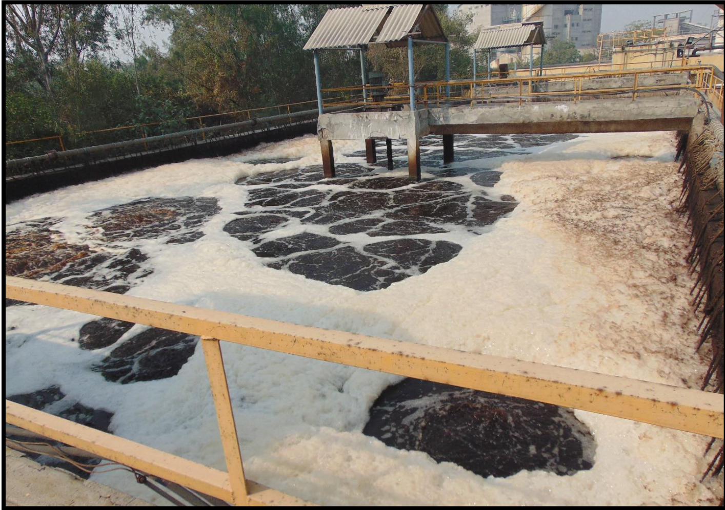
Figure 3.4 Industrial scale aeration tank-2
