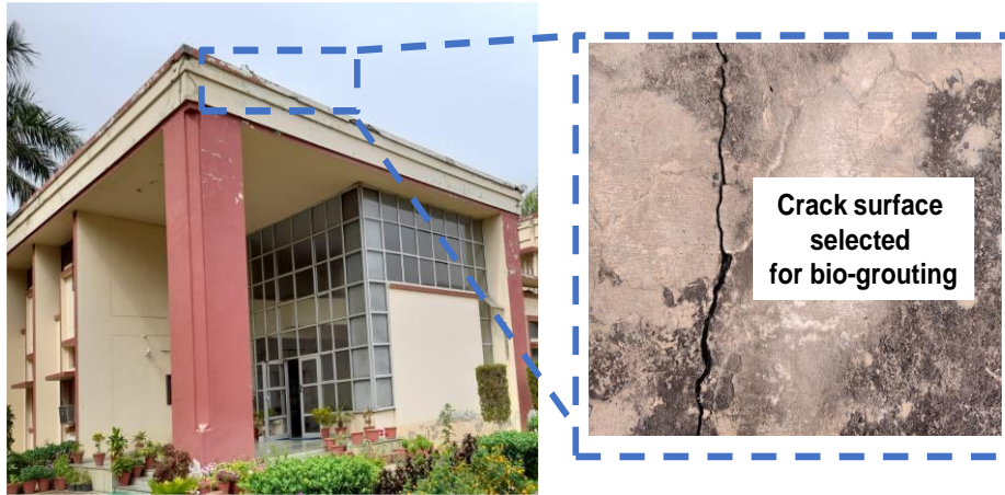
Figure 5.35: Identified damaged location for application bio-cementitious grout
